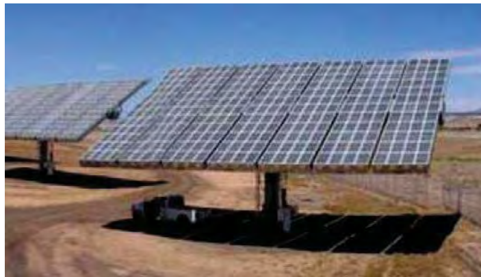
Canon Solar Partners proposes to use the 35 kW Amonix system (Canon 2008)
