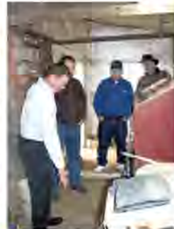
Greenhouse owner demonstrating wood chip boiler
