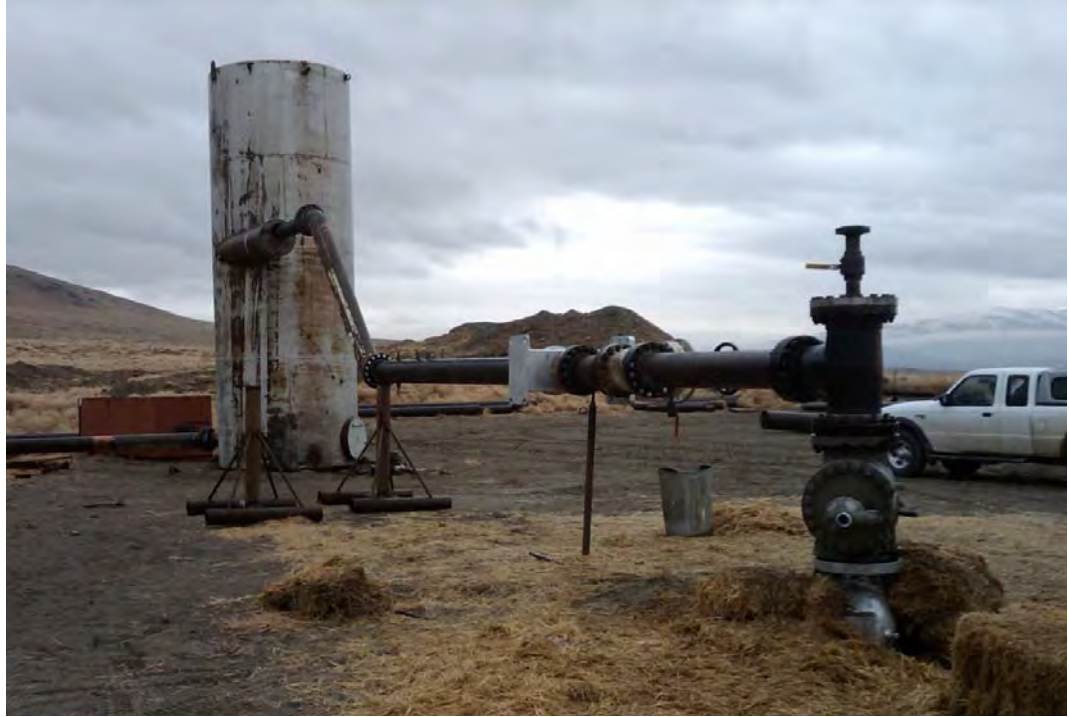
Figure 15: Wellhead, Flow Line, Control Valve, James Tube and Atmospheric Separator Used in a Geothermal Well Flow Test in Nevada, Similar to, but Smaller Than the Separator to be Used At Newberry.
