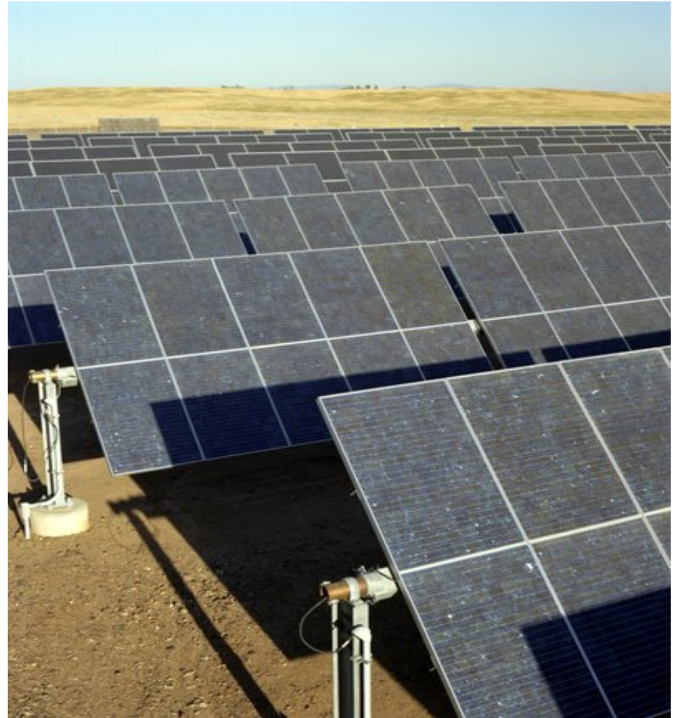
Photo by Warren Gretz, NREL
