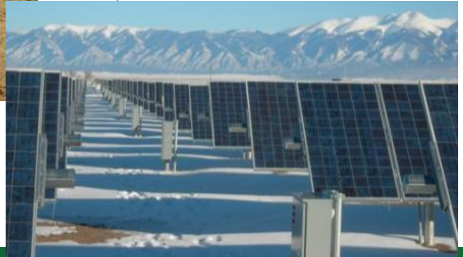
Alamosa PV System, Alamosa, Colorado Photo by Tom Stoffel, NREL
