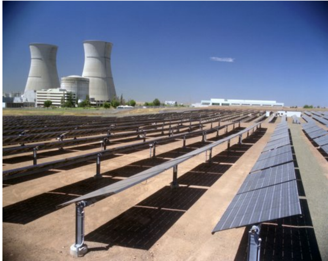
Photo by Warren Gretz, NREL
