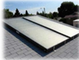
Solar Water Heating
