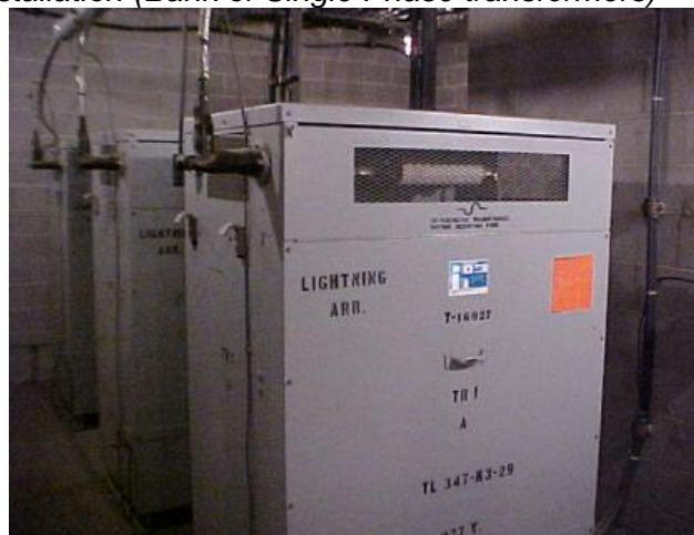
Dry type transformer installation (Bank of Single Phase transformers)
