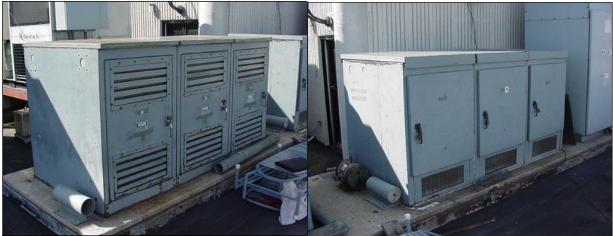
Rooftop dry type transformer installation
