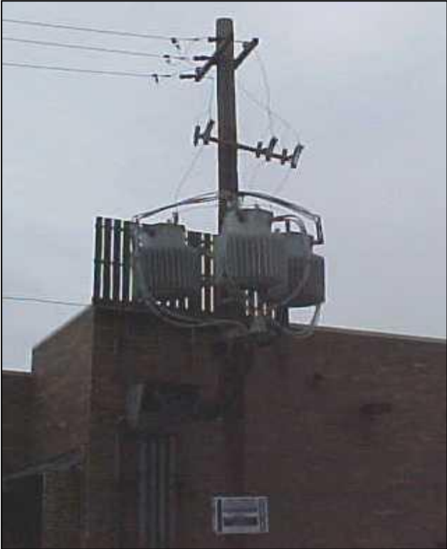
Pole 500kVA cluster mounted overhead transformers
