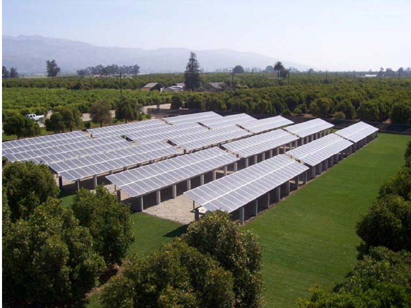
Photo: Travis Richardson, Hansen Trout Farm; Fillmore, CA. 105 kW California Solar Initiative Funded System, June 2007, Installer: GW Richardson Heating & Air Conditioning, Inc. Engineer/Designer: Kris Sutton, Travis Richardson
