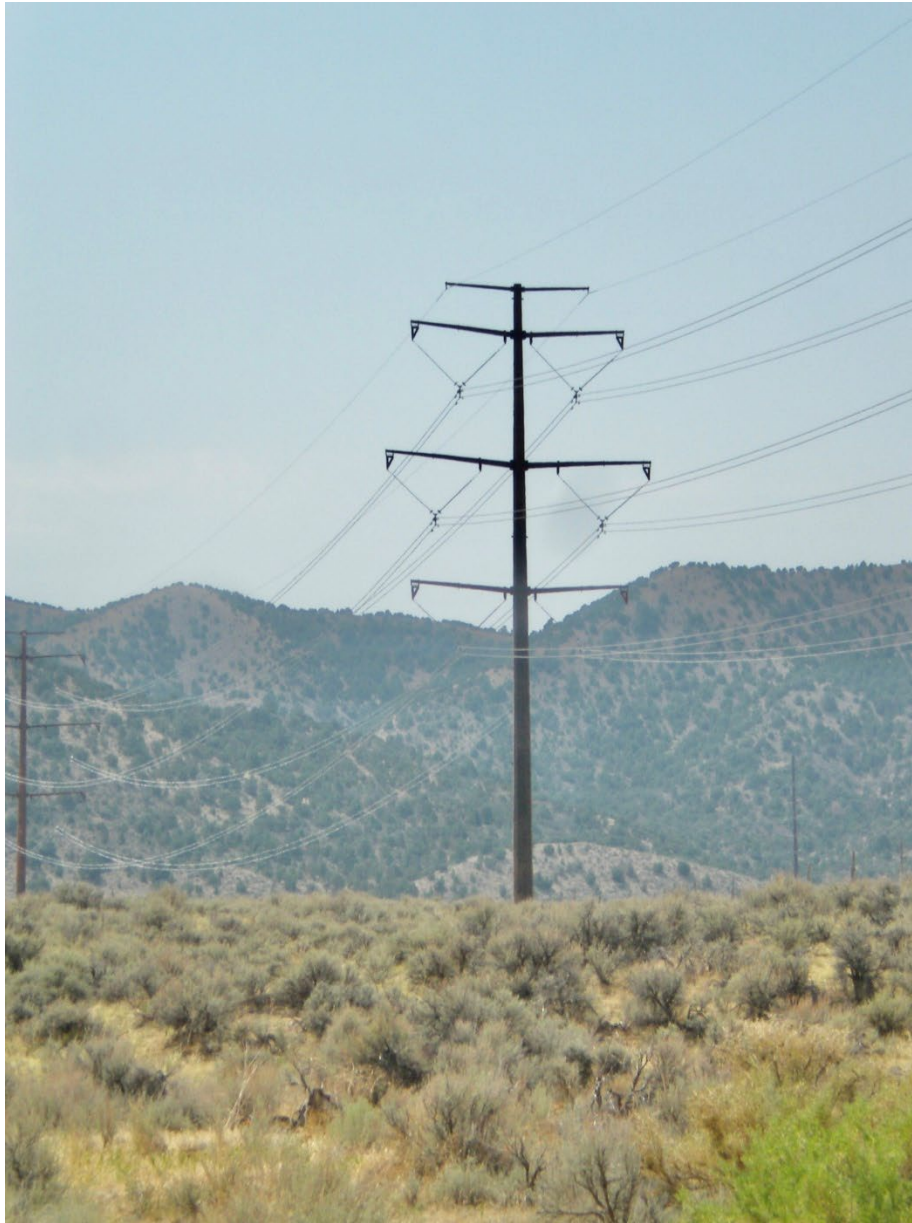
Figure 7. Image of Typical AC Monopole Structure
