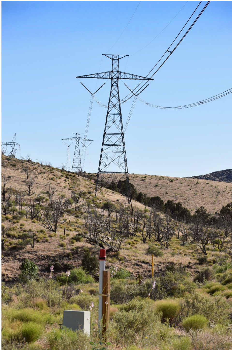
Figure 2. Image of Typical Steel Lattice Structure for HVDC Transmission
