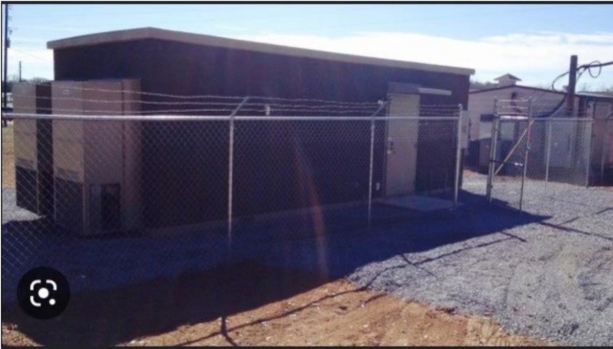
Figure 5. Images of Typical Optical Regeneration Facilities
