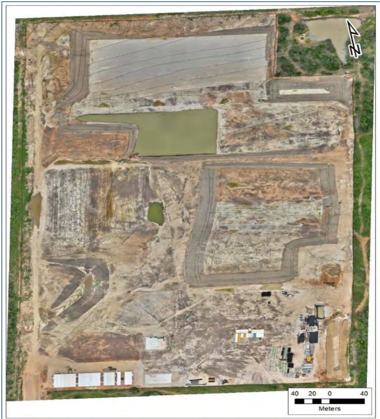
Figure 3a: Existing Conditions, May 2024, Project Site Main Facility – Cleared and Graded with Construction Staging Area and Temporary Stormwater Detention
