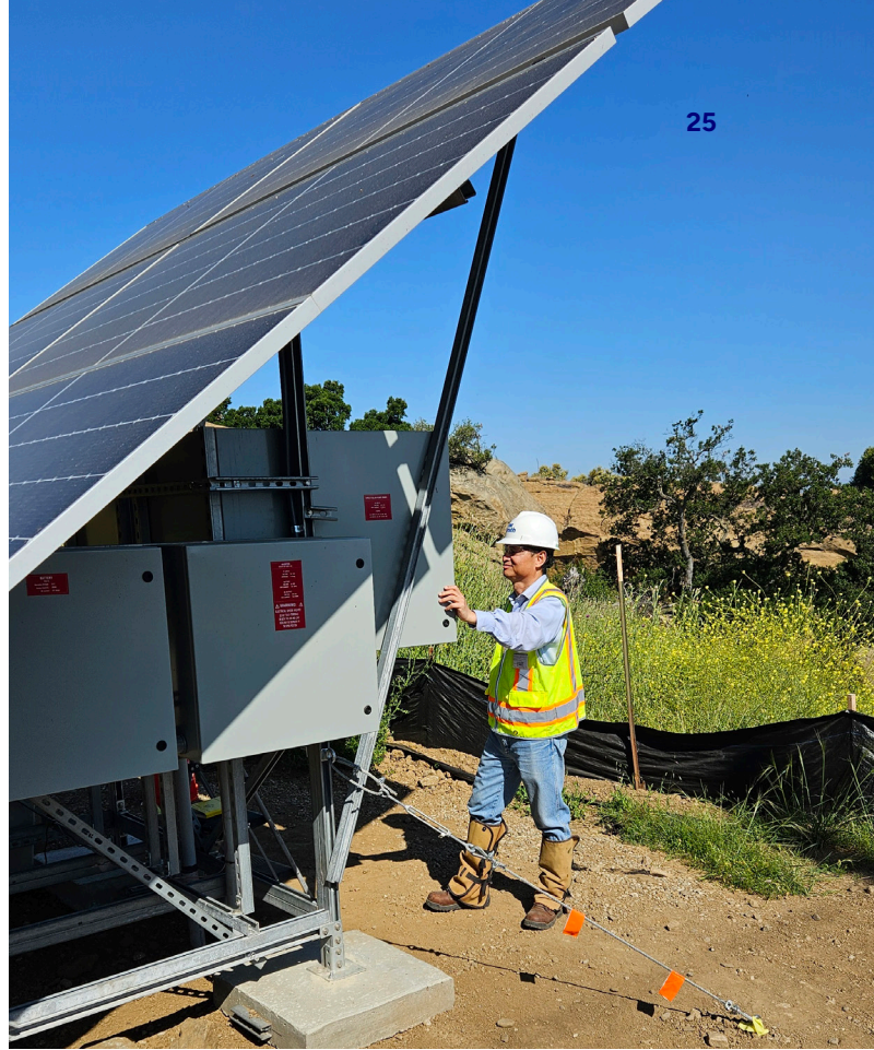
Workers check the solar skid panel and data on the human-machine interface software used for the automated groundwater interim measures project in Area IV at SSFL.
