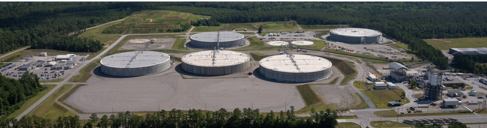
All major concrete placements have been completed on SDU 10 (far right); the latest mega-size disposal unit at SRS.
