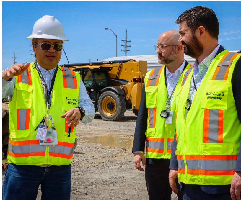
EM Principal Deputy Assistant Secretary Jeff Avery (right) and other EM officials tour the Portsmouth Site with the deactivation and demolition contractor.
