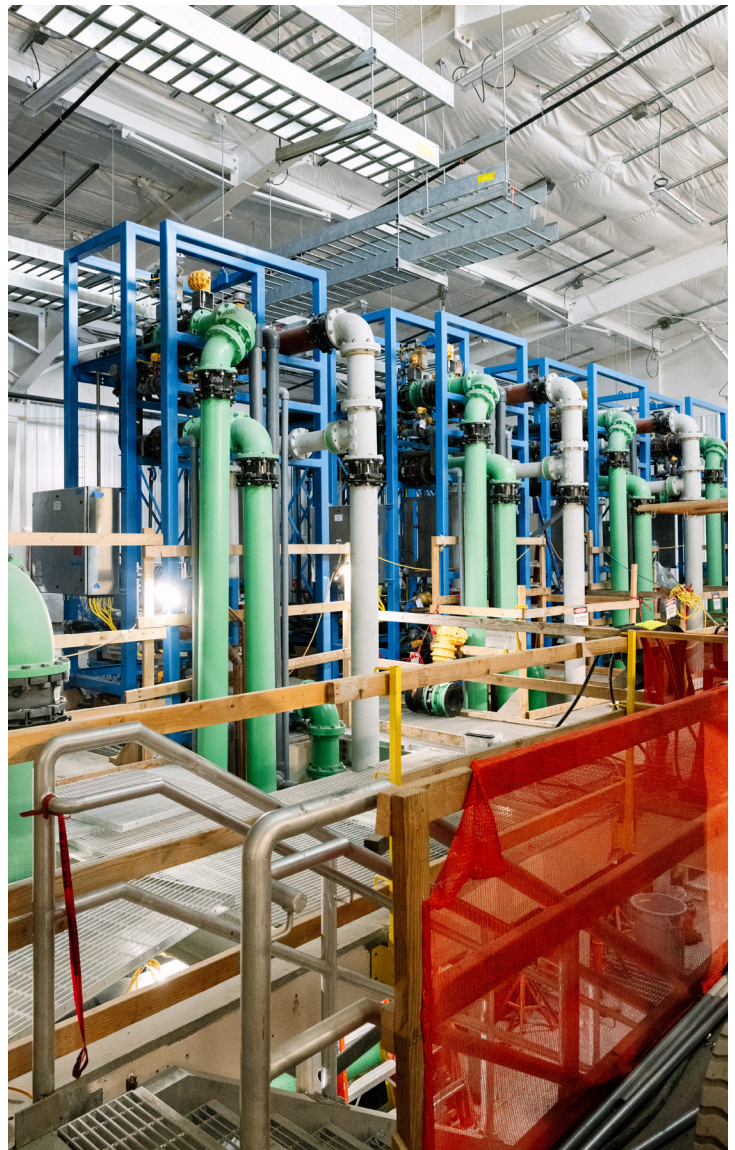
A glance inside the Central Plateau Water Treatment Facility shows construction progress.
