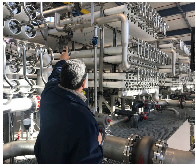
Plant Superintendent Art Ruiz points to the rows of reverse osmosis modules that can produce up to 27.5 gallons of fresh water for the city of El Paso, TX. This facility is the site of pioneering pilot studies supported by NAWI to transform the waste brine from the desalination process into valuable industrial chemicals. Photo courtesy of Pete S. Fiske, Director of the National Alliance for Water Innovation
