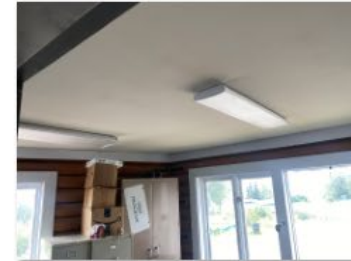
(Tribal Center) New office light fixtures
