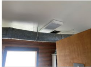
(Tribal Center) Mens bathroom new light fixture
