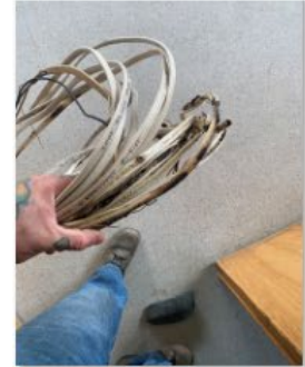
(Tribal Center) Old burnt wiring from trough fixtures
