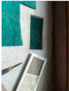
(Tribal Center) Return air register filter
