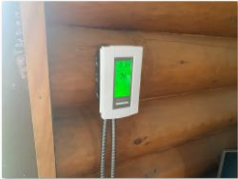
(Tribal Center) Meeting room new thermostat
