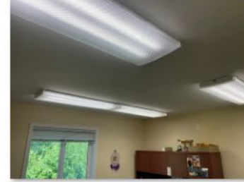
(Corporation Office) Office 1 Lighting
