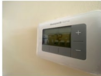
(Corporation Office) Replaced Thermostat
