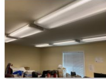
(Corporation Office) Office 2 light fixture
