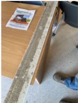
(Tribal Center) Old troughs light fixtures
