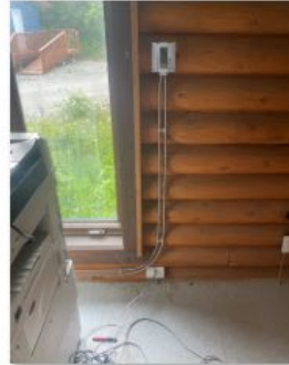
(Tribal Center) New baseboard heater thermostat
