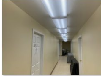
(Corporation Office) Hallway Lights
