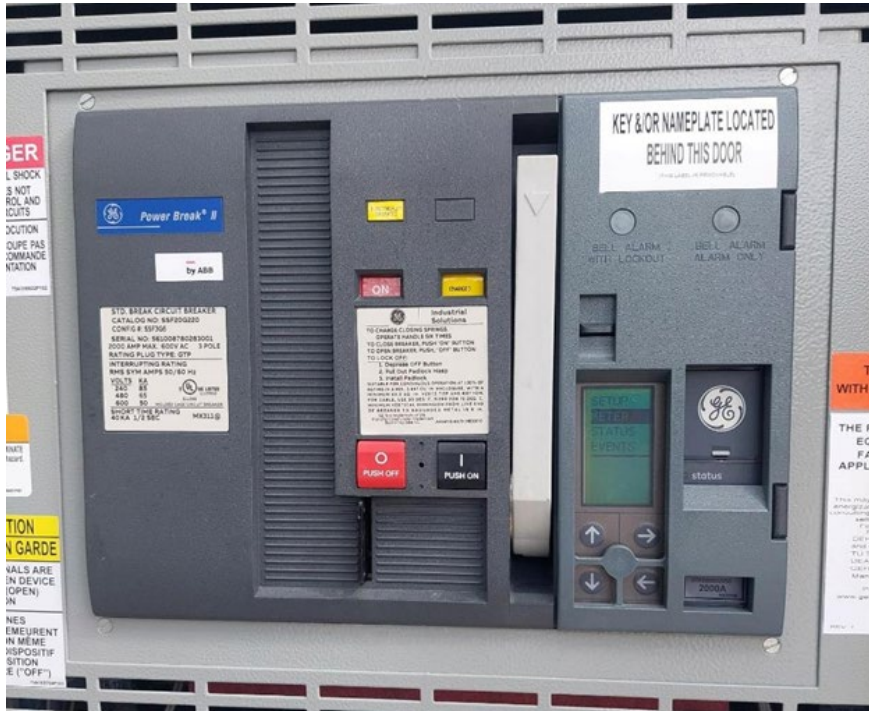
Motorized Breaker missing UPS backup
