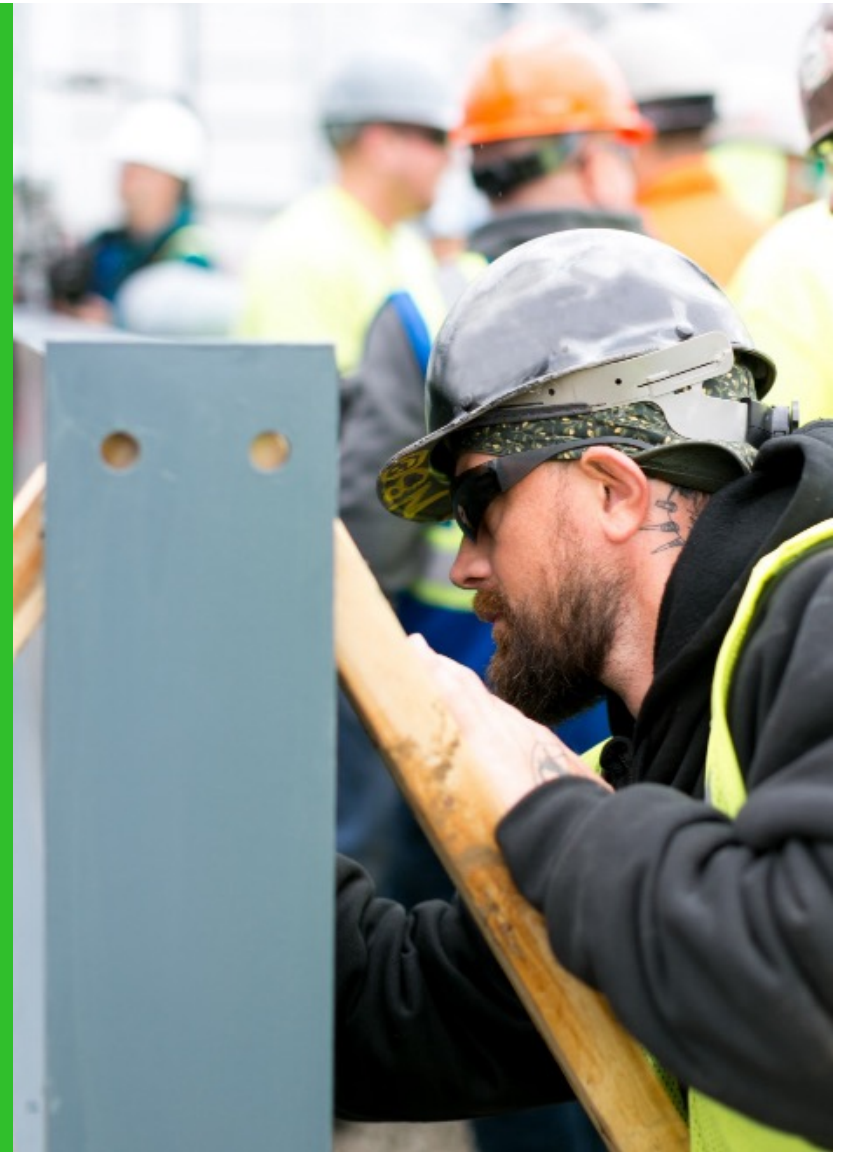
▲ Crews signing the last beam to be put into place at Cirba Solutions' lithium-ion processing facility expansion in Lancaster, Ohio. (Image courtesy of Cirba Solutions).
