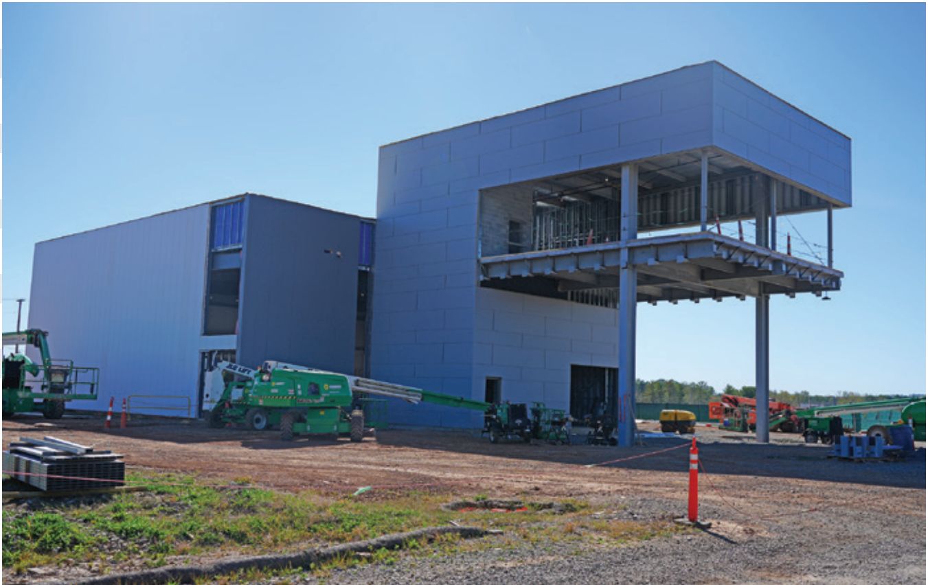
A lot of construction progress on the viewing platform was made in FY 2024
