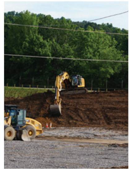
Remediation at one of the EUs, EU-17. Below, the EU-21 team, which was tasked with the largest remediation subproject at ETPP
