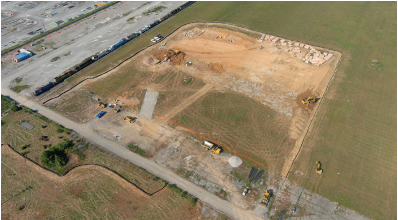
Kairos has begun construction of the Hermes Low-Power Demonstration Reactor at ETTP
