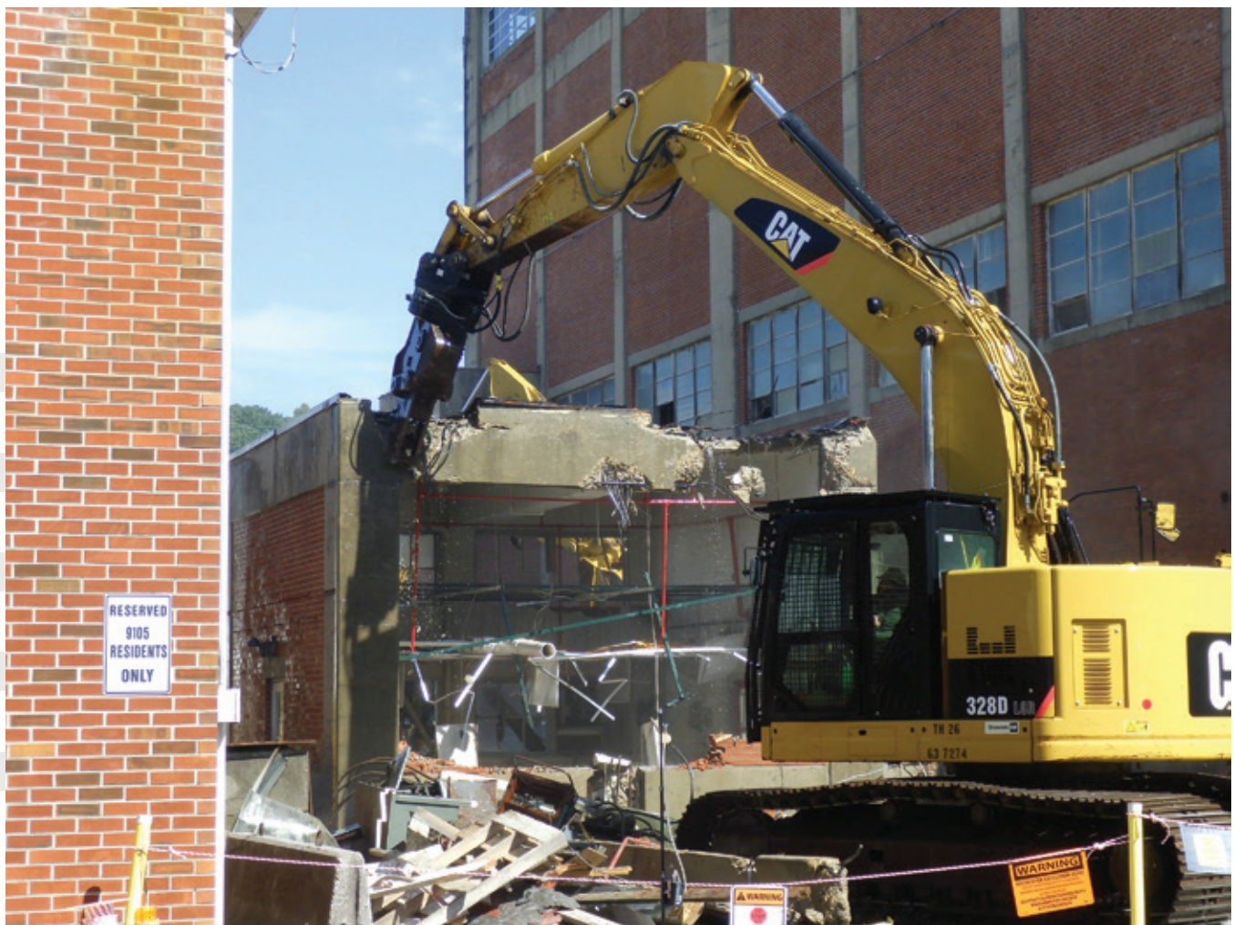
Demolition of the Alpha-2 Complex begins with removal of the carpentry shop
