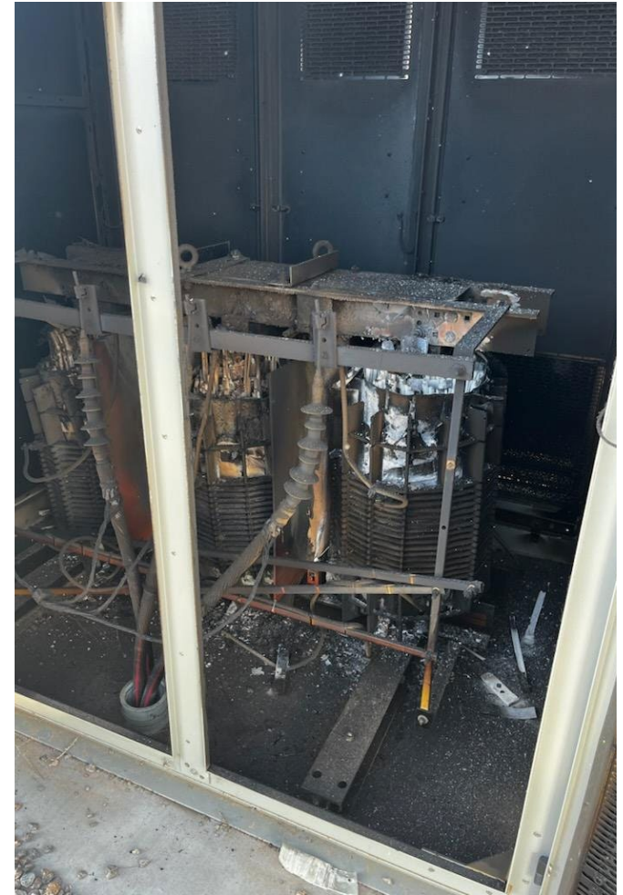
Picture of Interior of Zig-Zag Transformer taken a day after the fire.
