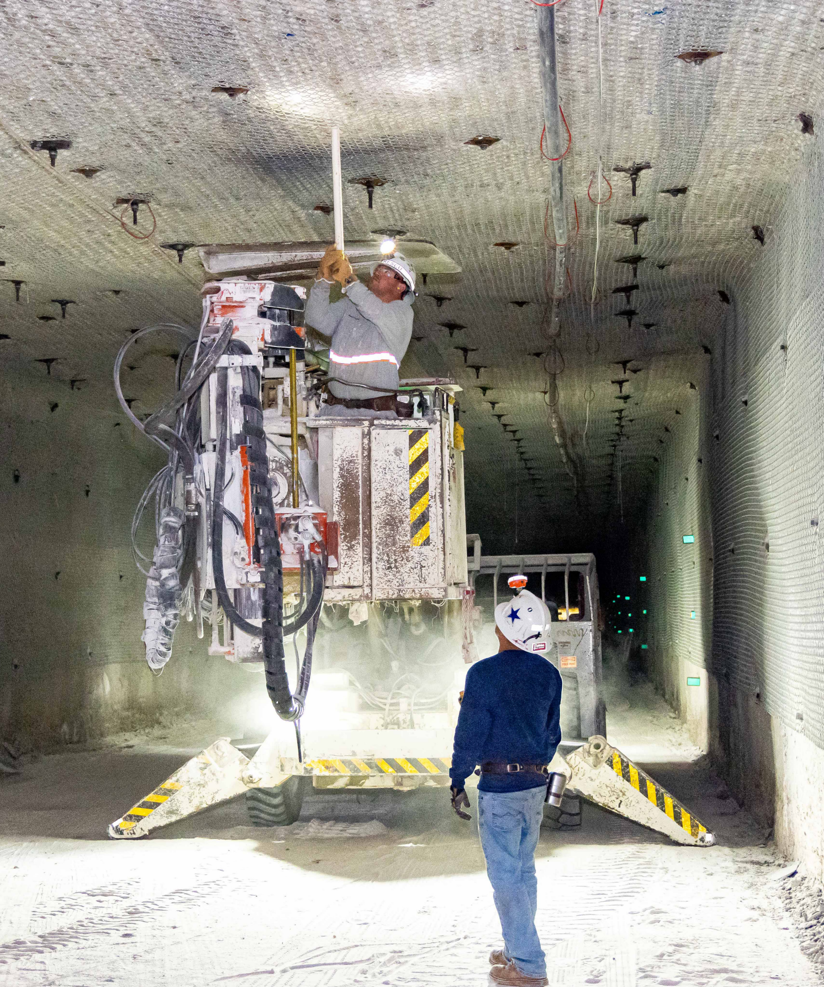
Workers install reinforcement bolts into the "back" or ceiling of the mined ancient salt bed in the WIPP underground. The salt formation creeps slowly, so the bolts hold the back of the mined rooms where TRU waste will be emplaced.
