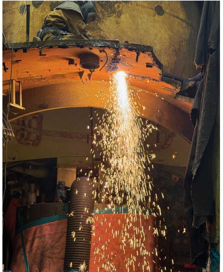
A worker uses a plasma torch to cut through a hull at the S1W prototype.
