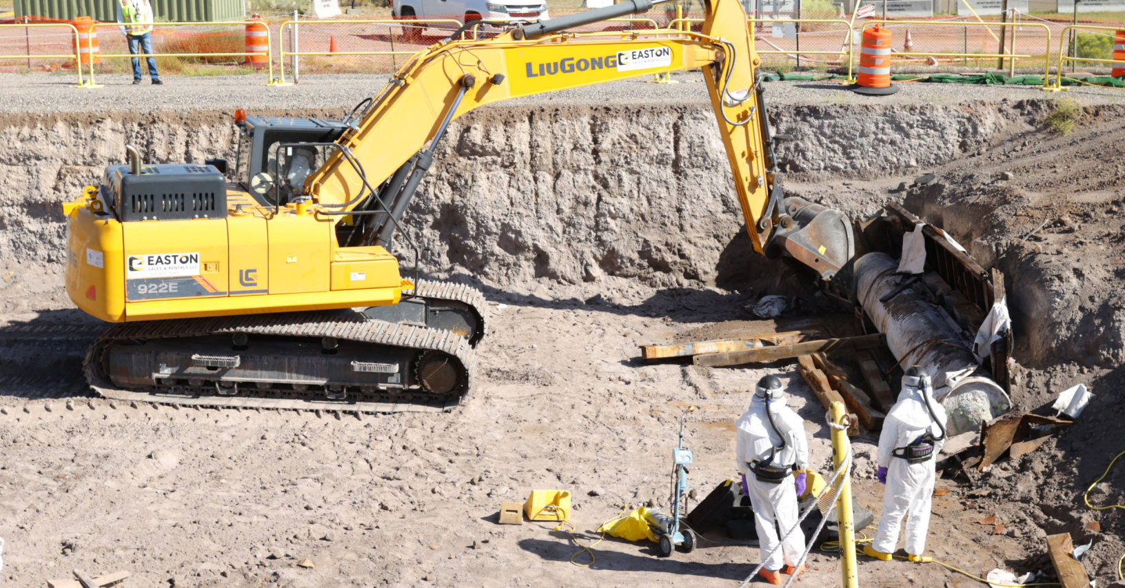
Waste Operations workers retrieve the final corrugated metal pipe containing cemented TRU waste at TA-54, Area G.
