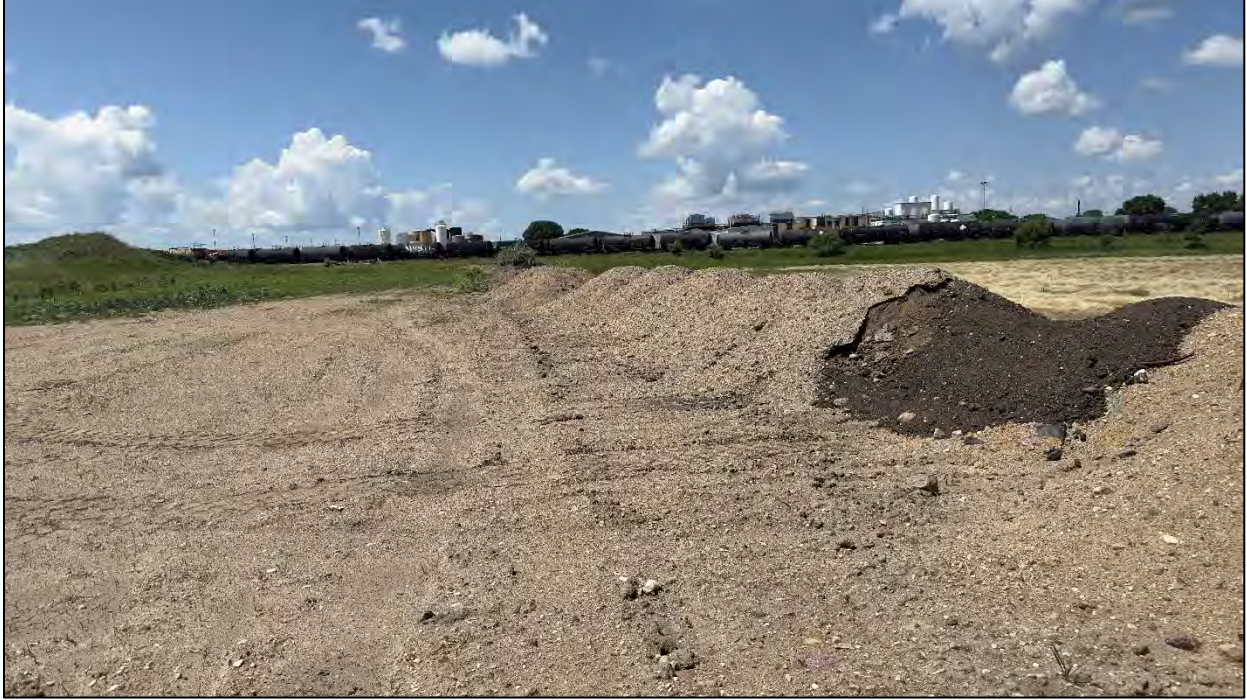
Photograph 7: earthwork activities along the southern portion of the Project area, view West.
