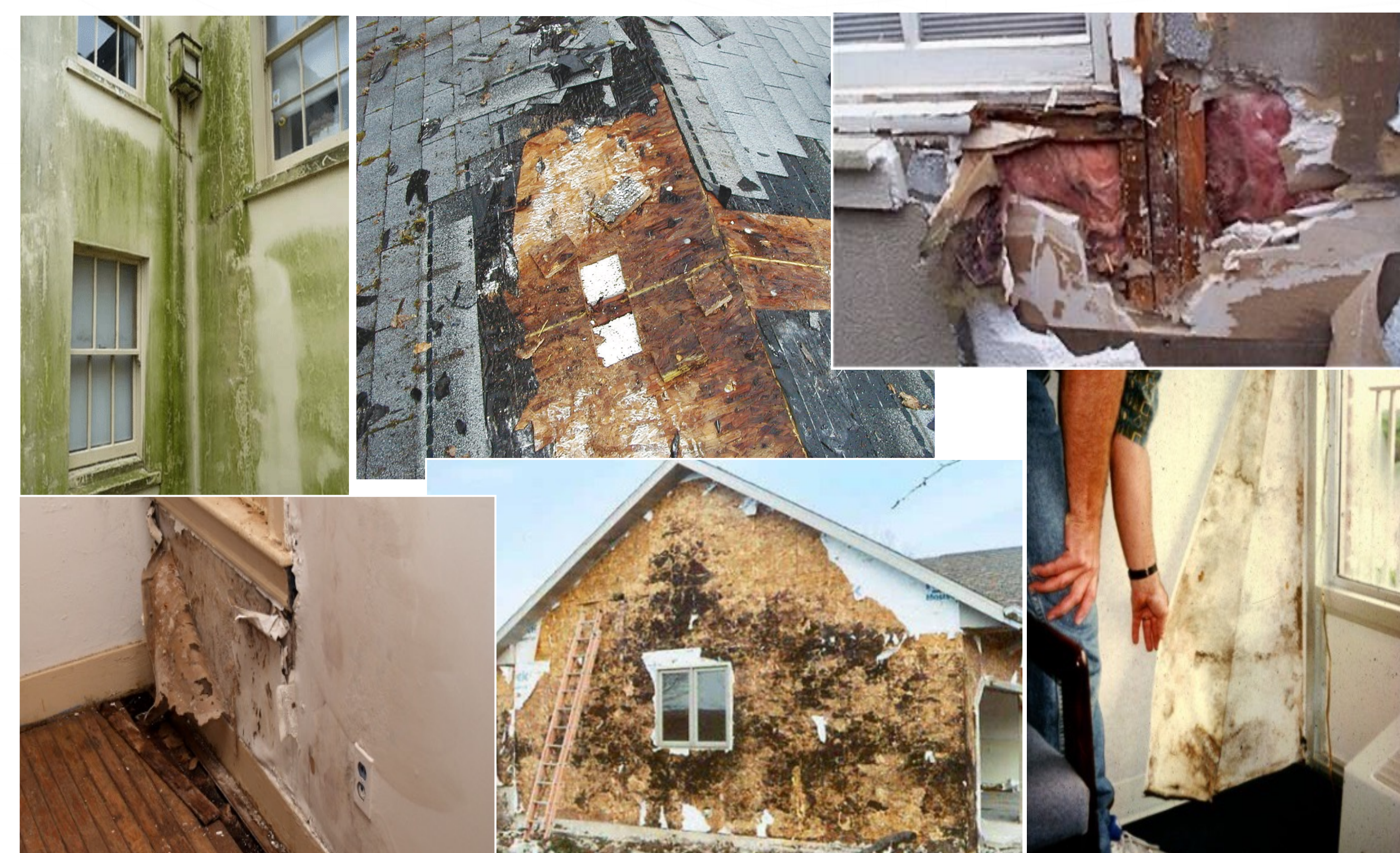
Mold, corrosion, wood rot, insect infestation, staining, algae, poor indoor air quality, and reduced energy efficiency are all performance problems created by moisture.
