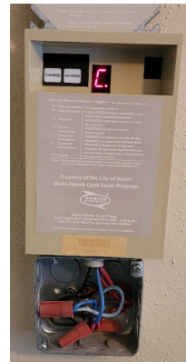
Legacy Water Heater Timer
