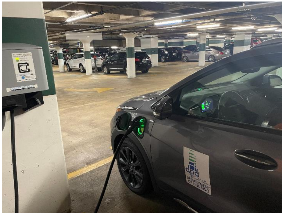
Figure I.24.2 A Chevrolet Bolt EUV owned by the Shelby County Department of Housing charges at the new Level 2 charging station installed at the Vasco A. Smith County Administration Building. Source: Memphis-Shelby County Division of Planning and Development.
