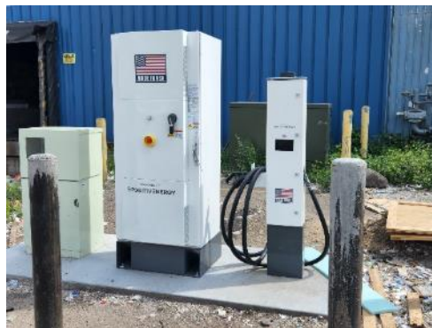
Figure I.19.5 Positive Energy DCFC
