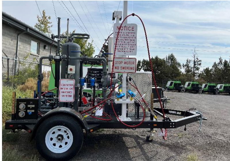
Figure I.38.2 Factory commissioned fueling station awaiting shipping in Bend, Oregon
