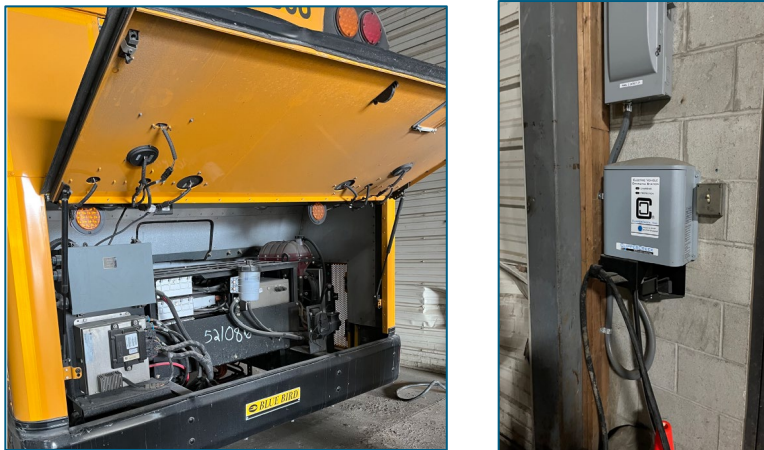
Figure I.19.3 Blue Bird bus battery compartment (left), Clipper Creek Level 2 charger (right)
