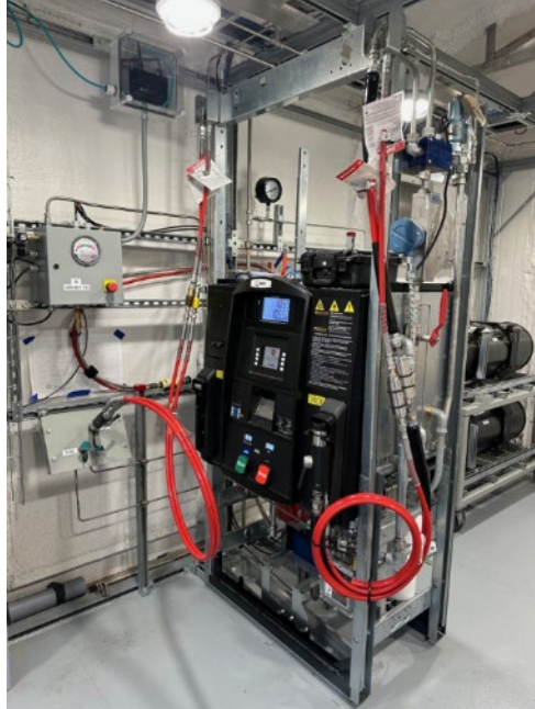
Figure I.5.2 The fully installed ANGI dispenser was moved into the test chamber along with two target cylinders.
