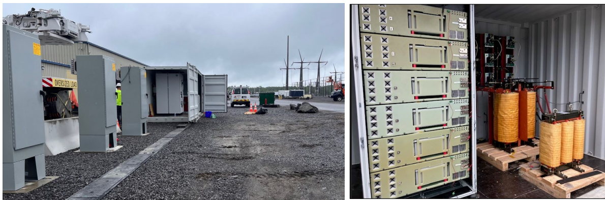
Figure II.1.13.7 Charger deployment at NYPA site. (Left) View of system installation with three DC/DC nodes, shipping container and Trenwa trench housing the DC cables. (Right) View inside the container showing DC connection.
