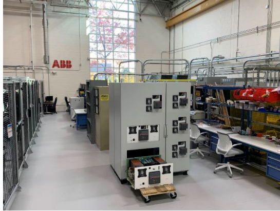
Figure II.1.13.4 ABB switchgear after testing at ABB and prior to shipping to NCSU.
