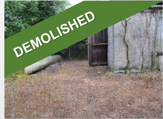
C-611-Q Raw Water Line Booster Station
