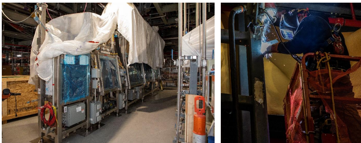
Equipment installation in the Main Process Building (left) and a worker in the Salvage and Accountability Building (right) at the Y-12 Uranium Processing Facility in 2023
