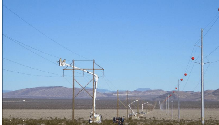
Crews working on the 138 kV Power Transmission System Replacement Project at NNSS
