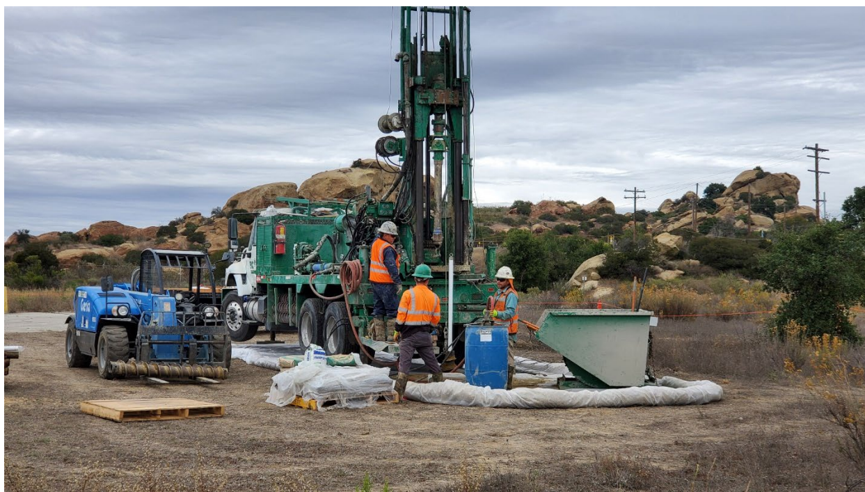
Figure 1. Installation of New Monitoring Wells in the Hazardous Material Storage Area (photograph taken November 15, 2023)
