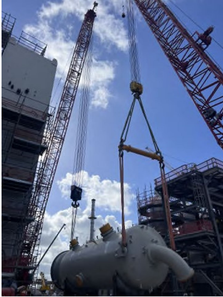
Photo 2: Train 2 Mixed Refrigerant Suction Drum
