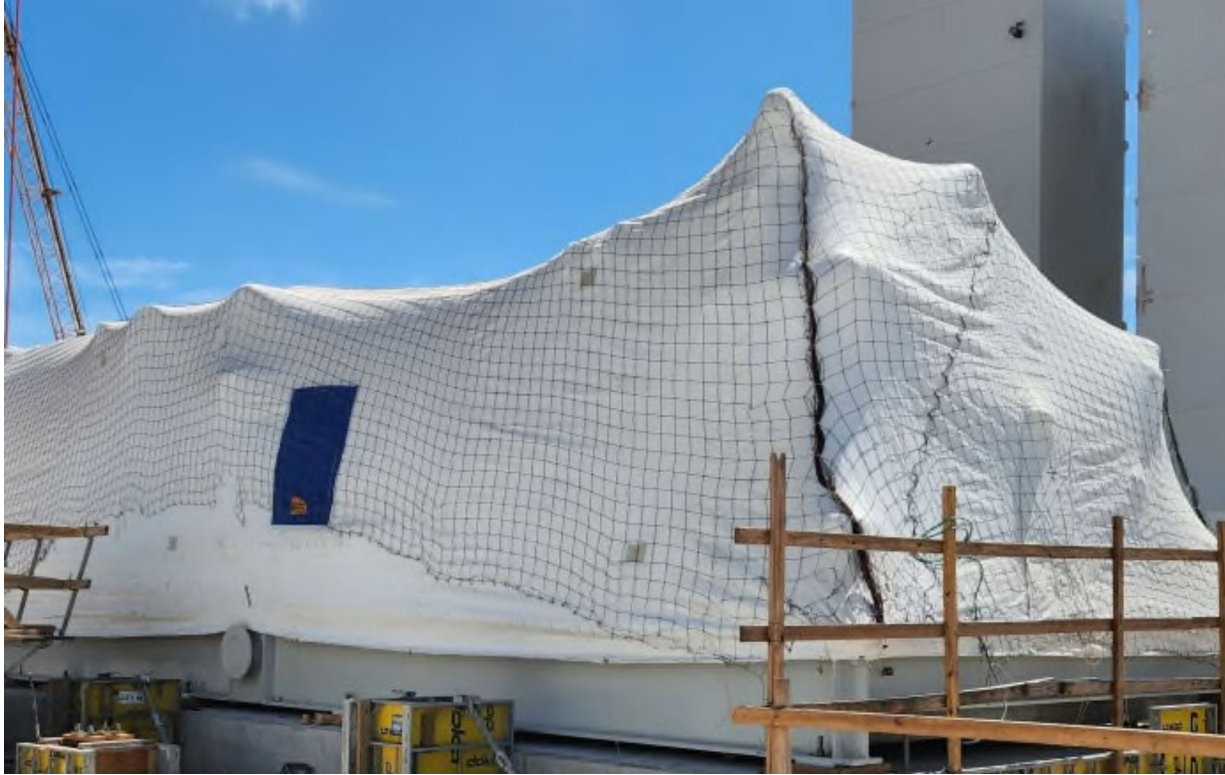
Photo 2: Train 5 Mixed Refrigerant Compressor
