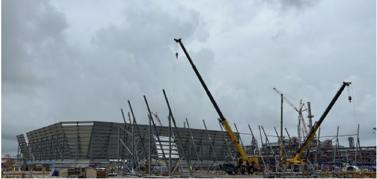
Photo 1: OSBL East Ground Flare 1
