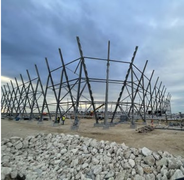
Photo 1: 310M01 Ground Flare 1 Steel Divider
