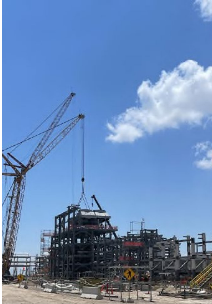
Photo 3: Train 2 AGRU Air-Cooled Heat Exchanger Set
