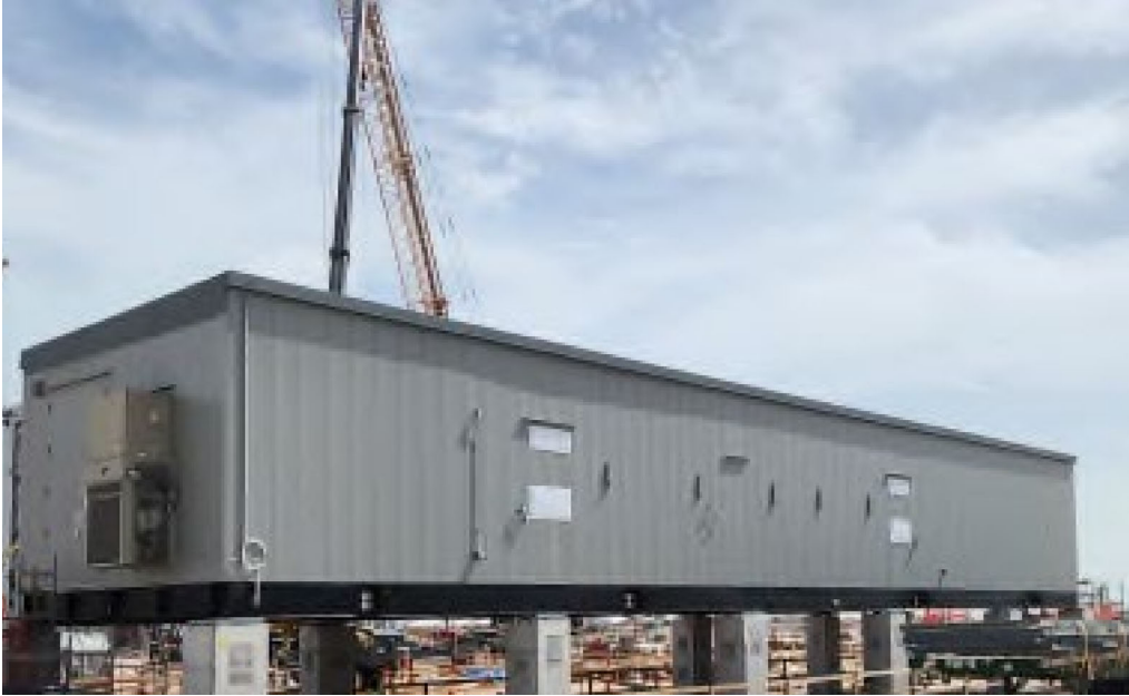
Photo 4: Train 5 Utility Substation
