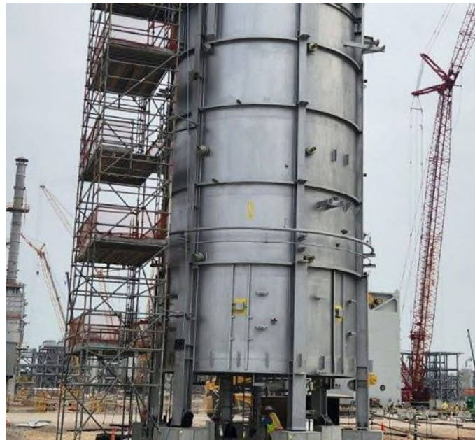
Photo 5: 344M01 Train 4 Hot Oil Furnace Set
