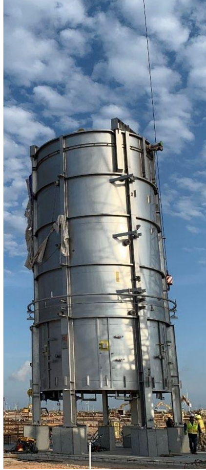
Photo 4: Train 6 Hot Oil Furnace Set
