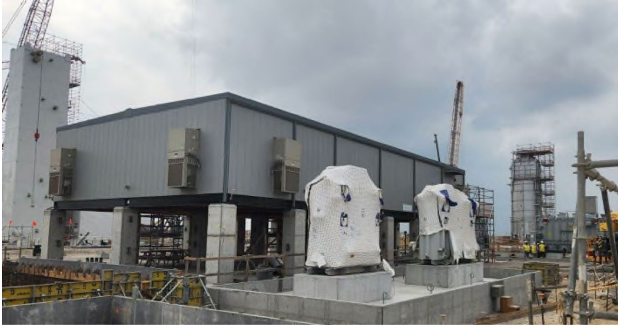
Photo 6: 333N01 Train 3 Liquefaction Substation Transformers Set
