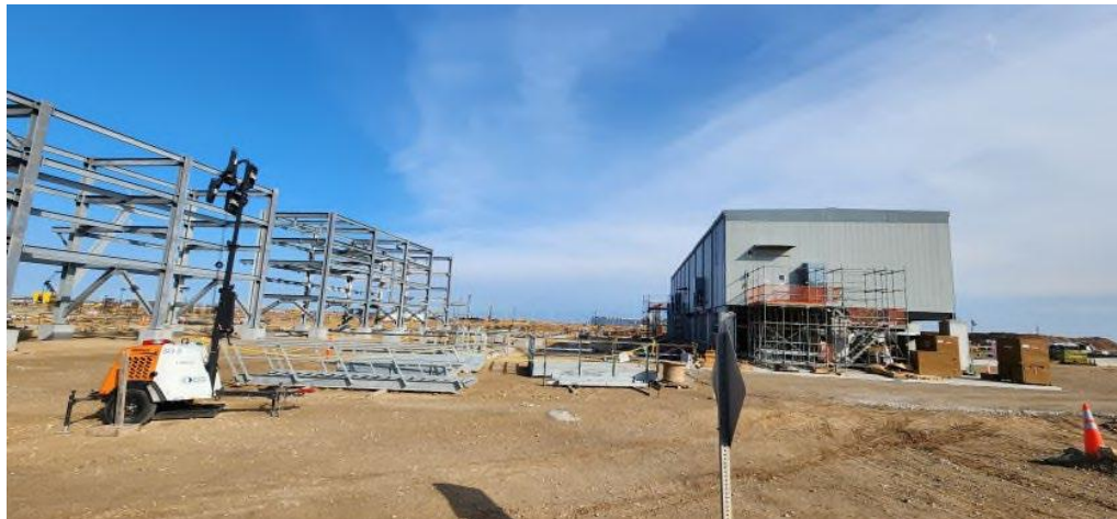
Photo 2: 310D01 GIS Substation Dress-Out
