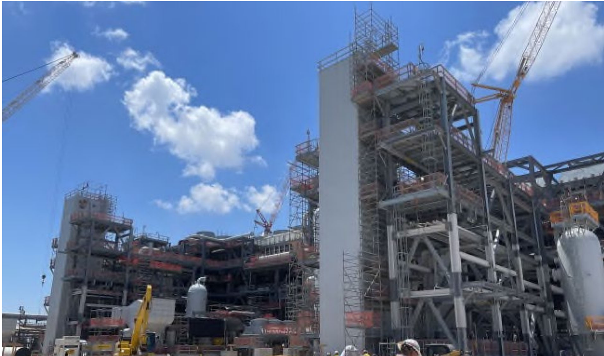
Photo 1: Train 1 Cold Box
