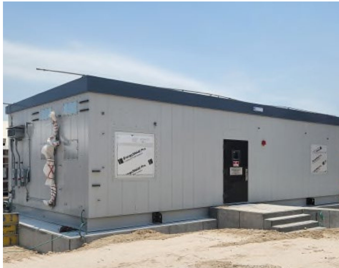
Photo 3: 310A01 OSBL South Operator Shelter Set
