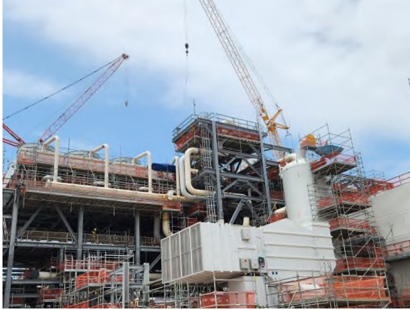
Photo 2: 311B01 Train 1 Air-Cooled Heat Exchanger Header Pipe
