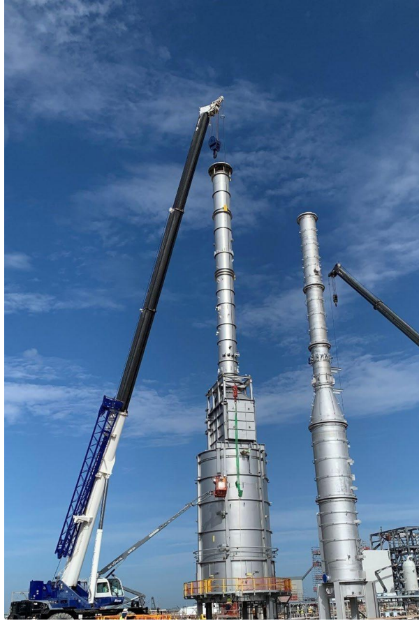
Photo 3: Train 4 Hot Oil Heater
