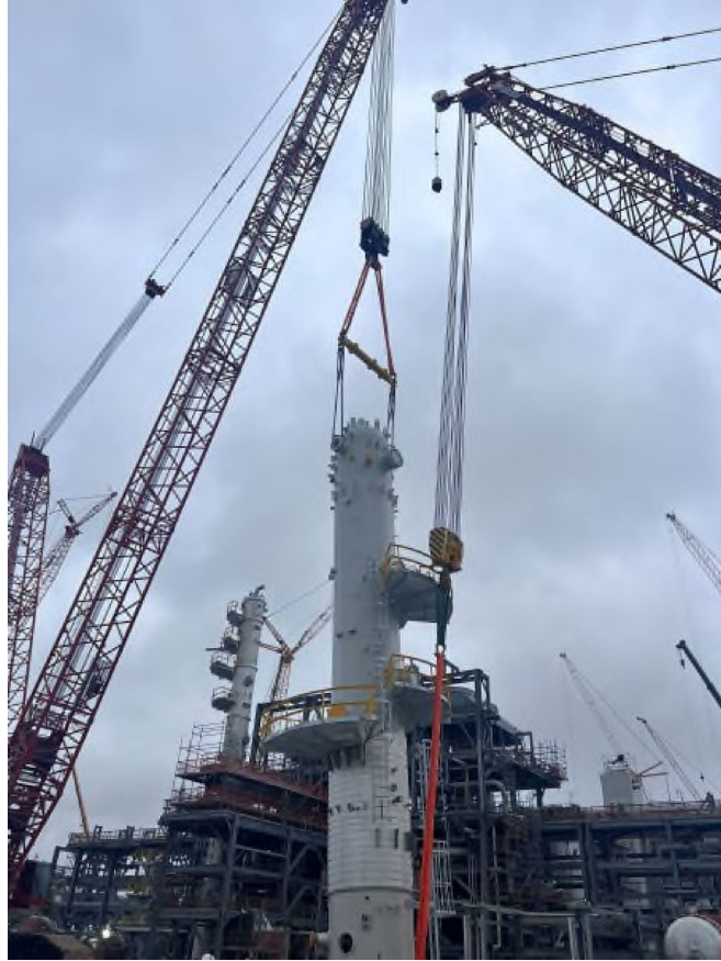
Photo 4: 311K01 Train 1 CO 2 Absorber Set
