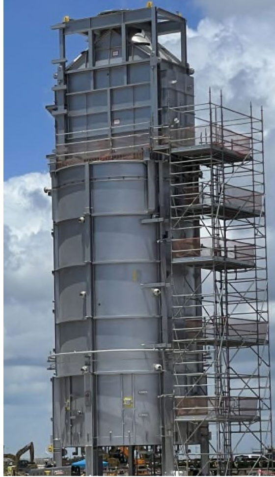
Photo 5: Train 5 Hot Oil Furnace
