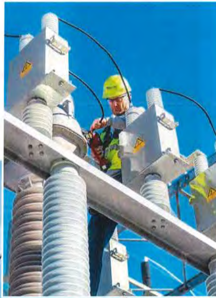
Jason Bjerke, senior technical maintenance technician, adjusts ripple injection equipment at the Wilton substation near Bemidji, Minn. The equipment is critical to Minnkota's demand response system.
