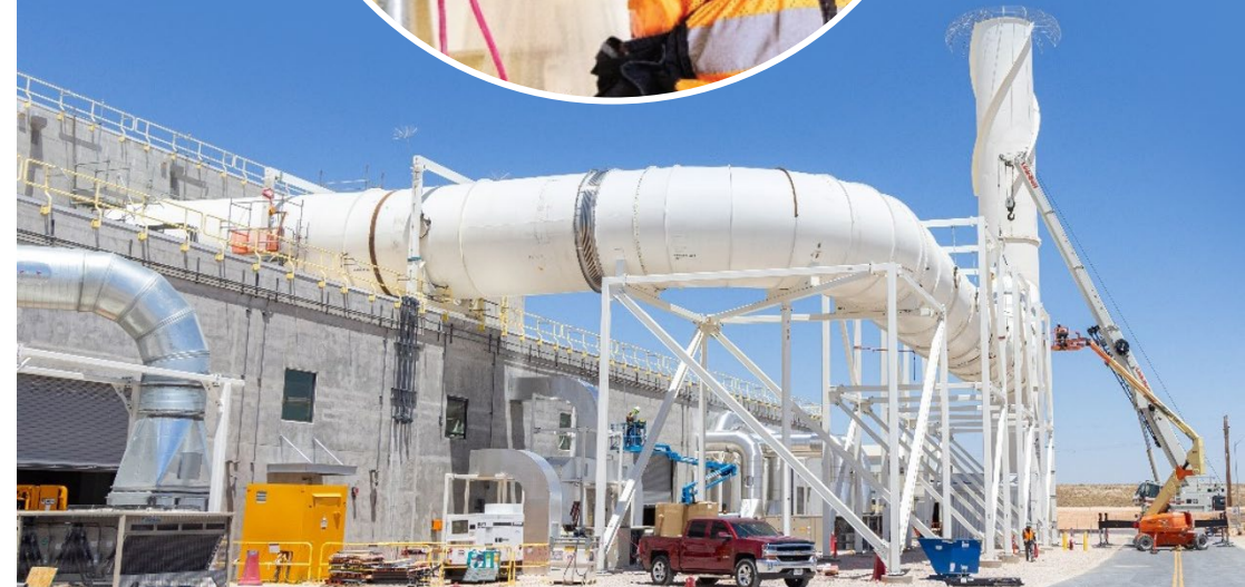
SSCVS final large ductwork installation
