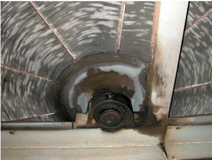
Wheel with Deformed Media Due to Lack of Glue
