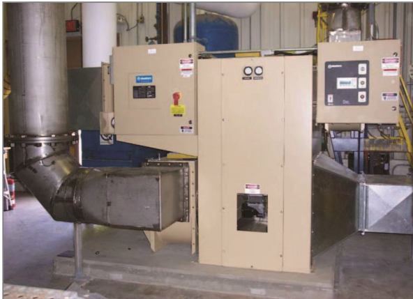
Ventilation of the underground HLW tanks by the Tank and Vault Drying System (T&VDS)
