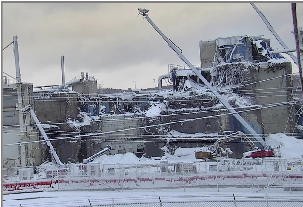
Deconstruction of the west side of the MPPB. The west side housed the CPC, COA, and MOA
