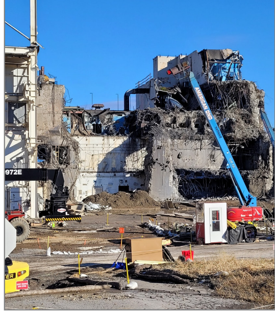
The MPPB deconstruction is conducted in a manner protective of on-site workers and off-site residents
