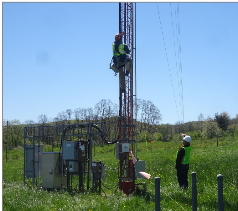
On-site meteorological monitoring tower undergoing inspection with oversight by the full-time on-site meteorological monitoring engineer
