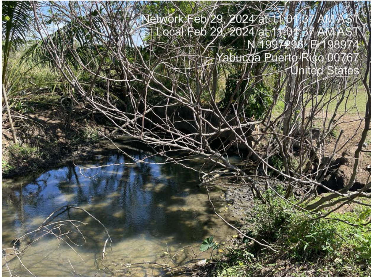
Picture 8 We also surveyed the crossings over the creek and irrigation channel.
