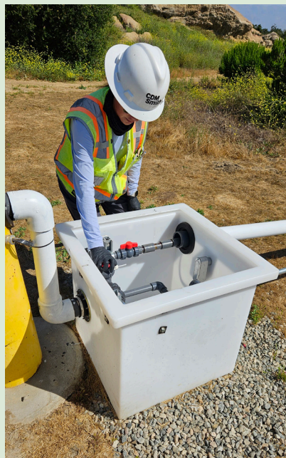
Sandra Ramos Hernandez with DOE contractor CDM Smith adjusts the control valve for automated groundwater extraction well C-24 in Area IV at SSFL. Photo courtesy of Song Chen.
