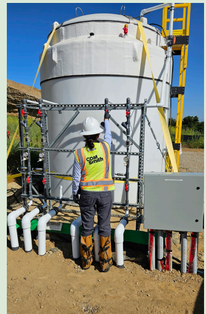
Sandra Ramos Hernandez with DOE contractor CDM Smith adjusts the ball valve on piping manifold located at the 5,000-gallon double-walled groundwater storage tank that was installed as part of the automated GWIM project in Area IV at SSFL. Photo courtesy of Song Chen.
