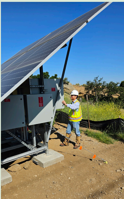
Song Chen with DOE contractor CDM Smith checks the solar skid panel and reviews data on the human-machine interface software used for the automated GWIM project in Area IV at SSFL. Photo courtesy of Sandra Ramos Hernandez.
