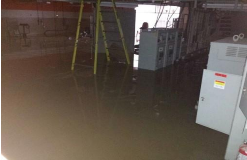
The rain flooded relay buildings in several critical 230kV stations in Toronto
