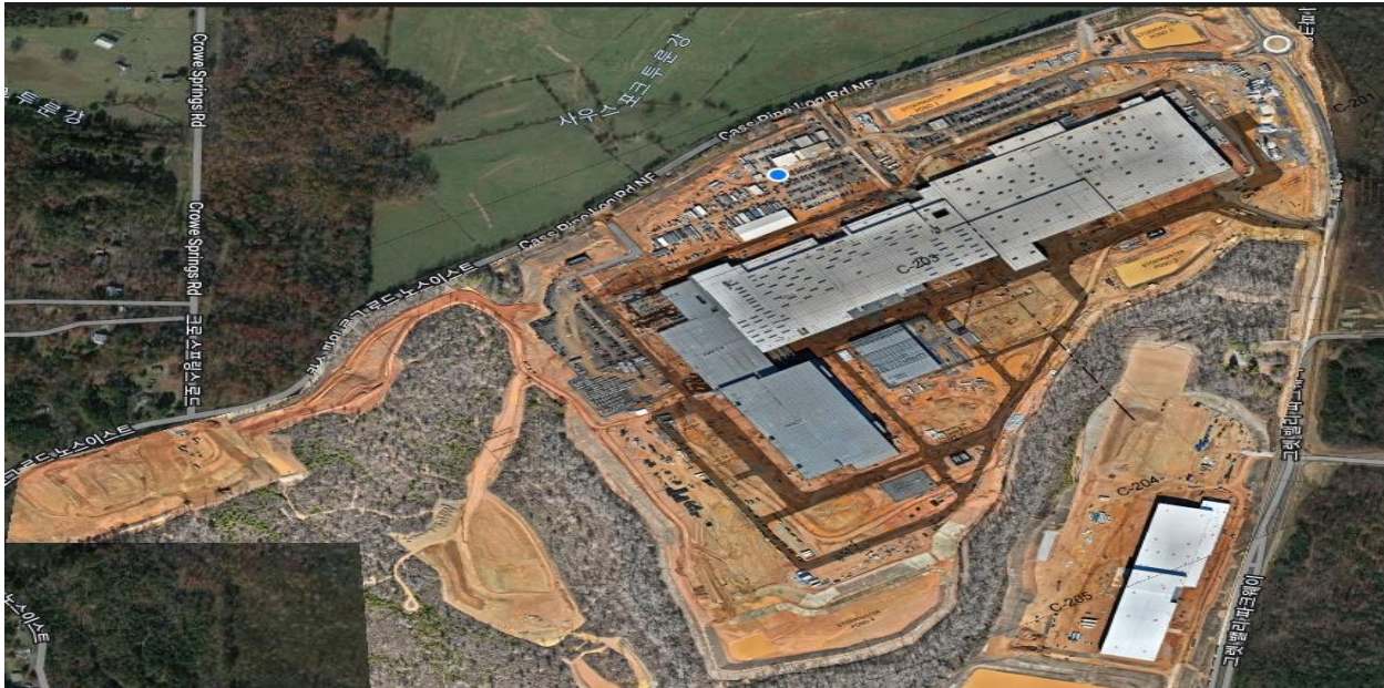
Exhibit 1-1. Overhead view of Project Redeemer as of January 31, 2024. The building at the bottom, right side of the image, and grading to the west are not associated with the Project.
