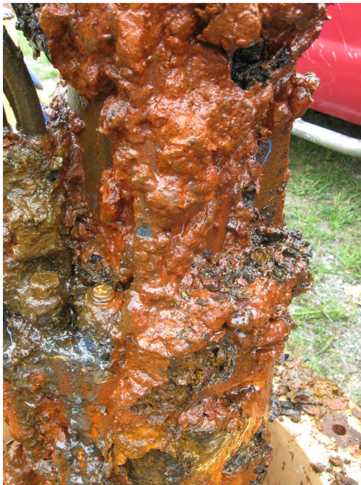
Figure A.1-4. Clean Pump (Top) Versus Iron-Fouled Pump (Bottom)
