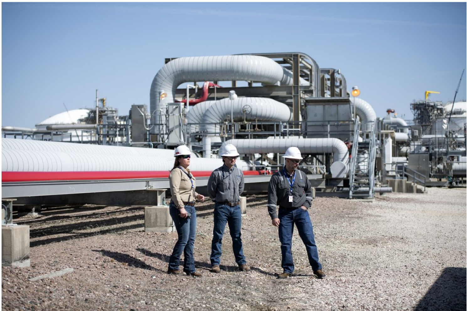
Workers at Cheniere Energy Inc.'s Sabine Pass LNG facility in Louisiana. Photographer: Mark Felix/Bloomberg
