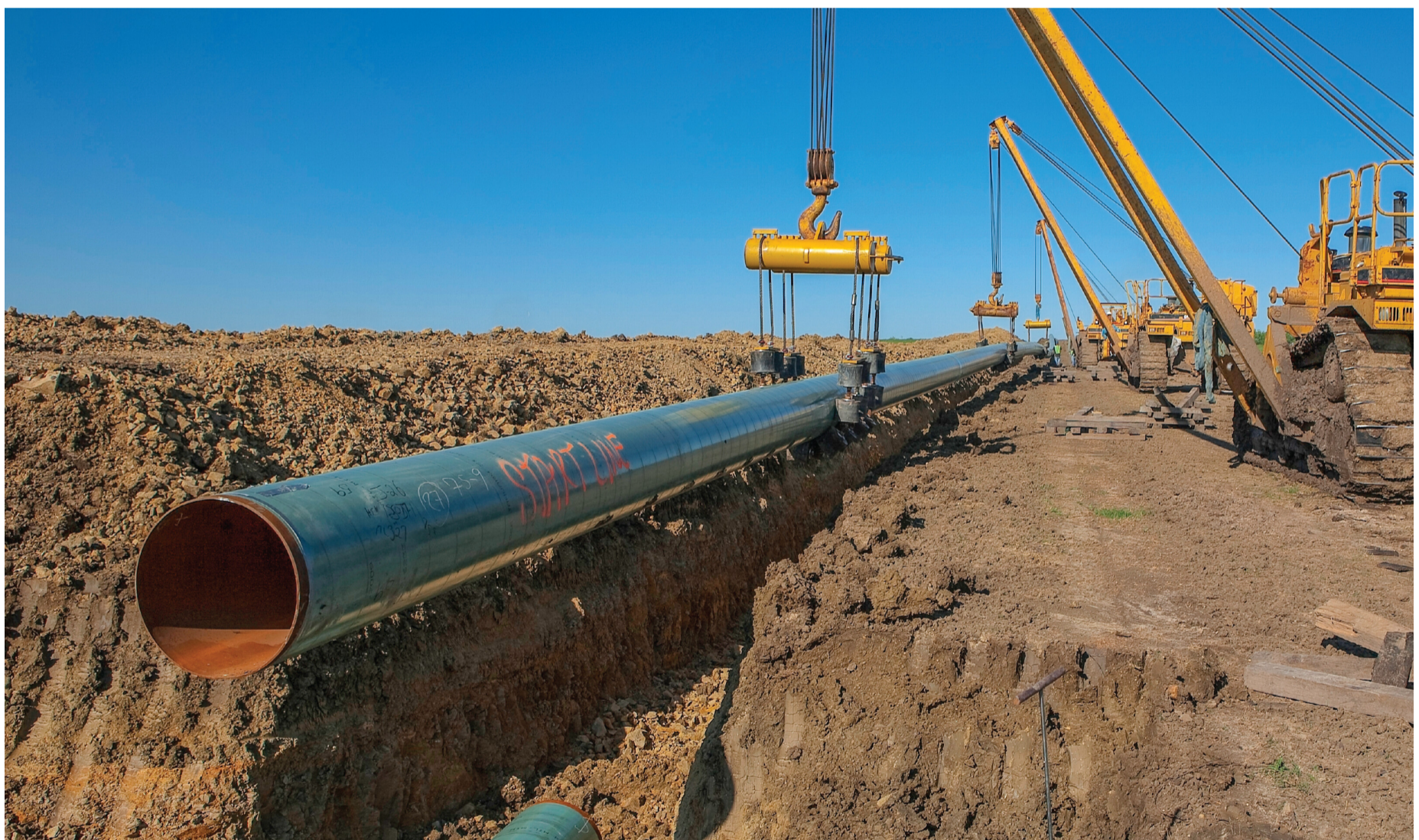
Pipe is laid during construction of a natural gas pipeline in Texas, USA. PHOTO: ED LALLO/GETTY IMAGES
