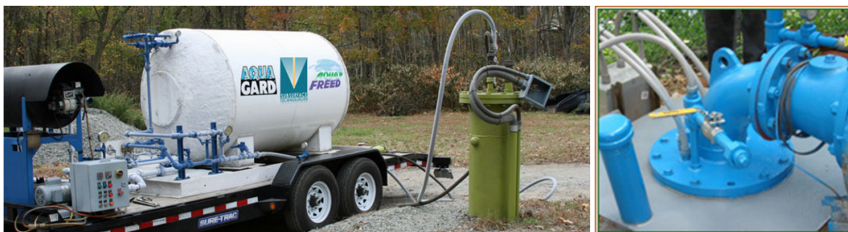
Photographs of Liquid CO 2 rehabilitation of a well and close up of deployment in well with pump remaining in place (courtesy of Subsurface Technologies, Inc. subsurfacetech.com)
