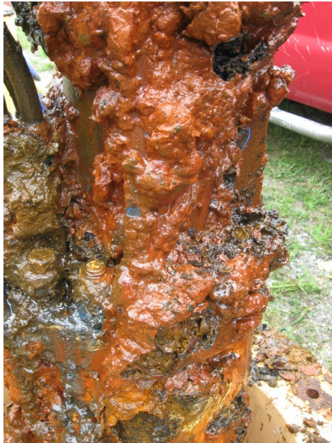
Figure 5. Clean Pumps (Top Photo) and Iron Fouled Pump (Bottom Photo)
