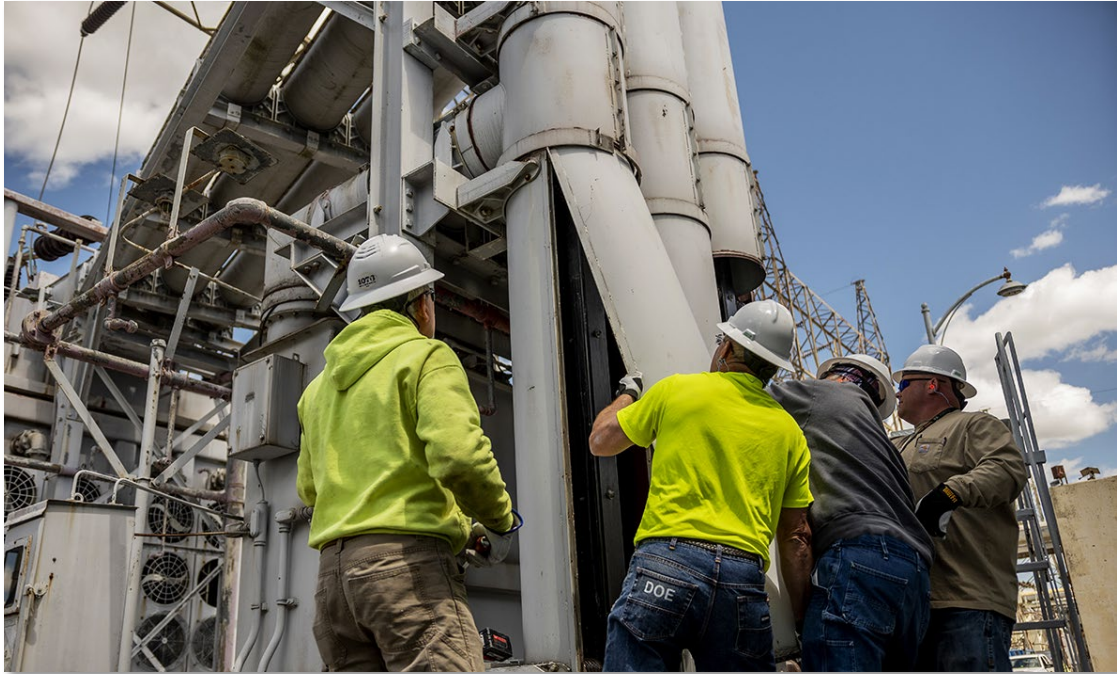
On May 1, 2023, casings surrounding Iso-Phase bus work are removed as crews begin work on the dismantlement of the C-535 switchyard.
