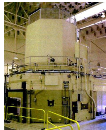
The B280 LPTR reactor vessel, pictured here in 2003, has been proposed for decommissioning.
