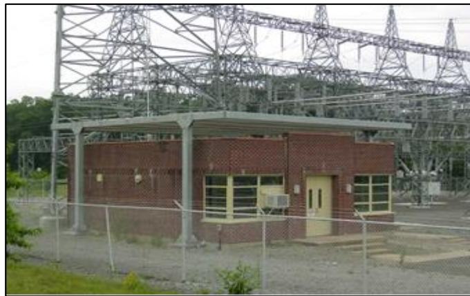
Figure 2 Van Buren Substation Control Building, Van Buren, Arkansas
