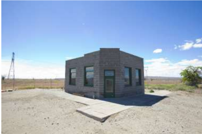
The exterior of the 1907 White Bluffs Bank in 2017, following DOE's rehabilitation work.
