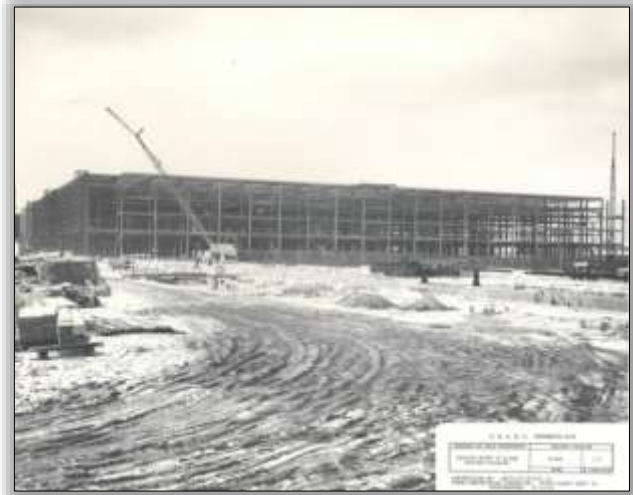
Northwest corner of the X-326 Process Building, facing southeast (building to be included in the HAER reports).
