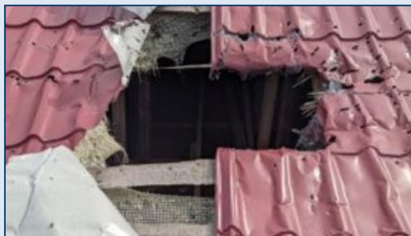
Damage to the roof of a facility housing radioactive sources as a result of Russian shelling.
