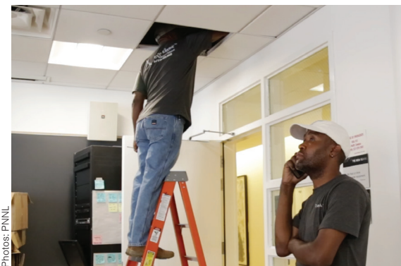
Installers placing LED fixtures in a classroom have their questions addressed by a manufacturer's representative on the phone.
