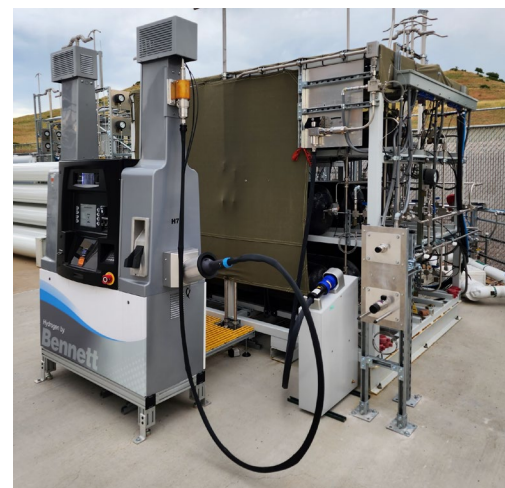
NREL and Bennett HD Dispensers
