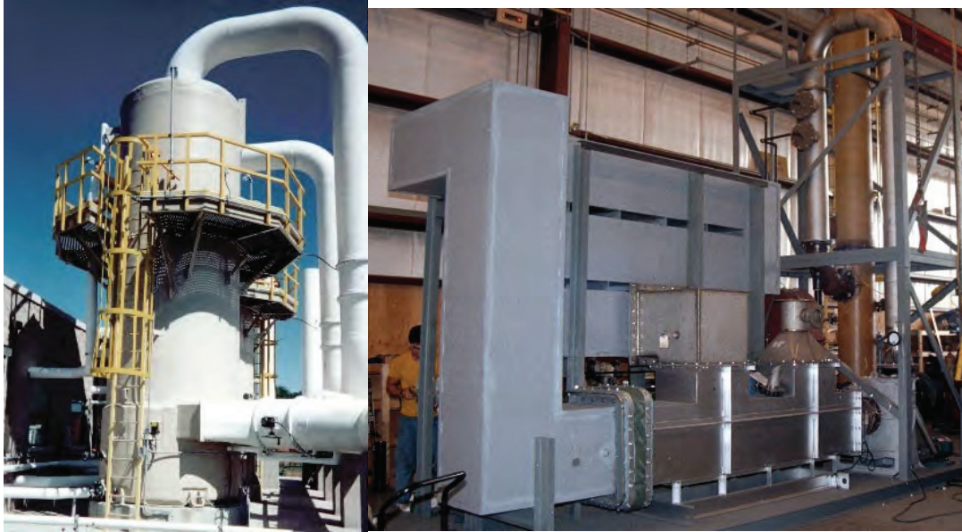
Figure 4. Commercial air stripping tower (left) and catalytic oxidizer (right).
