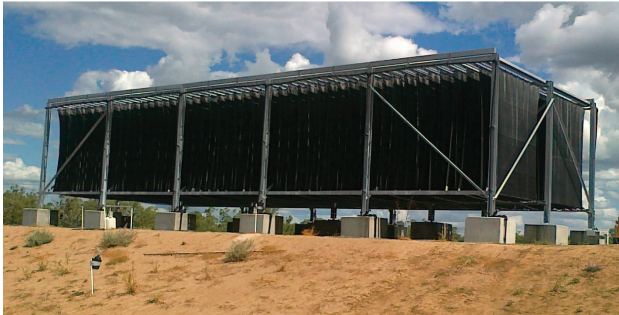
Figure 1. Installed WAIV system. Wind and enhanced evaporation is enhanced in a small footprint using large surface area panels.
