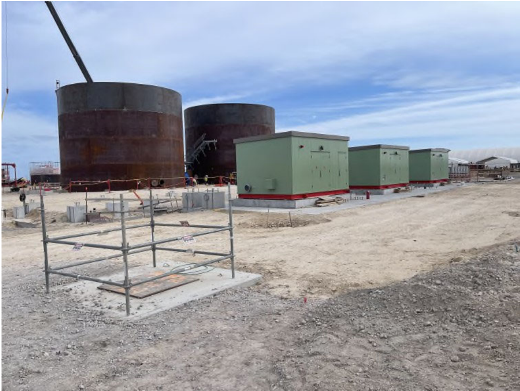
Photo 4: Area 310W01 OSBL East Firewater Pump Packages
