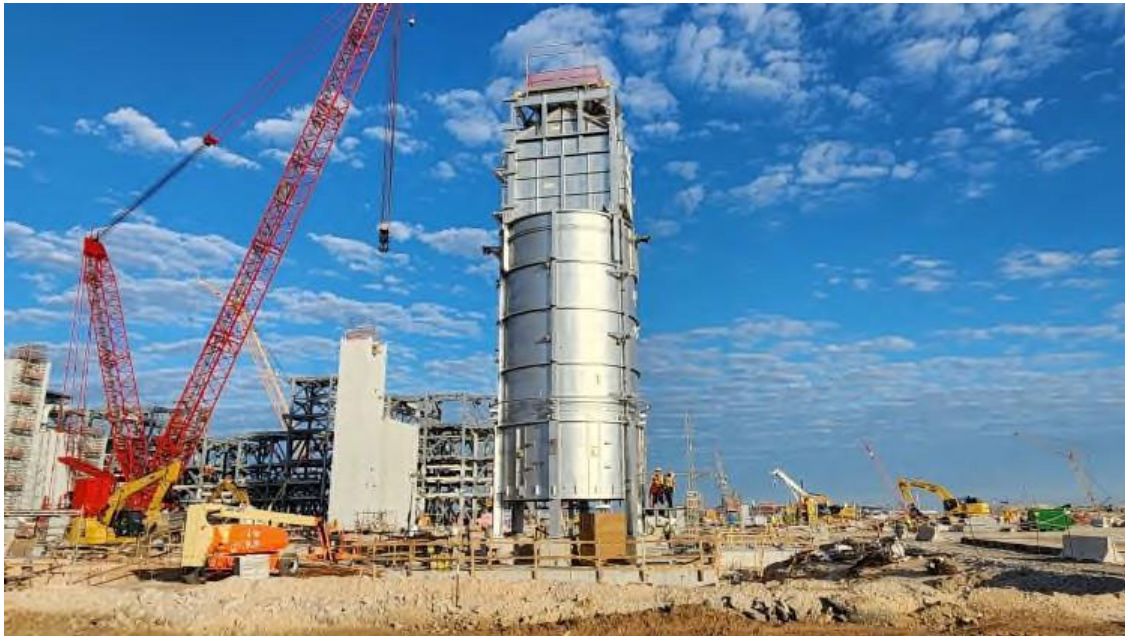
Photo 2: Area 311M01 Train 1 Hot Oil Furnace
