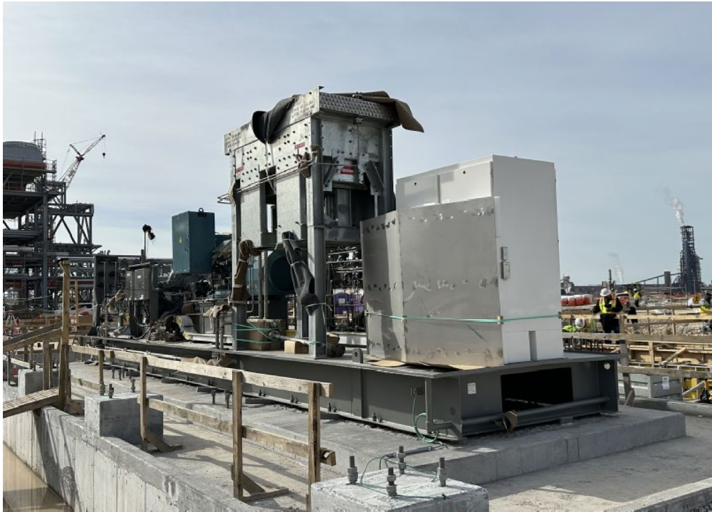
Photo 2: 322E01 Train 2 Regen Gas Compressor Set
