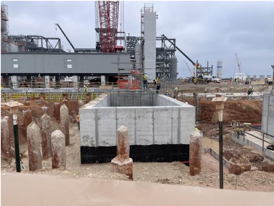
Photo 4: Area 311L01 Train 1 Amine Sump
