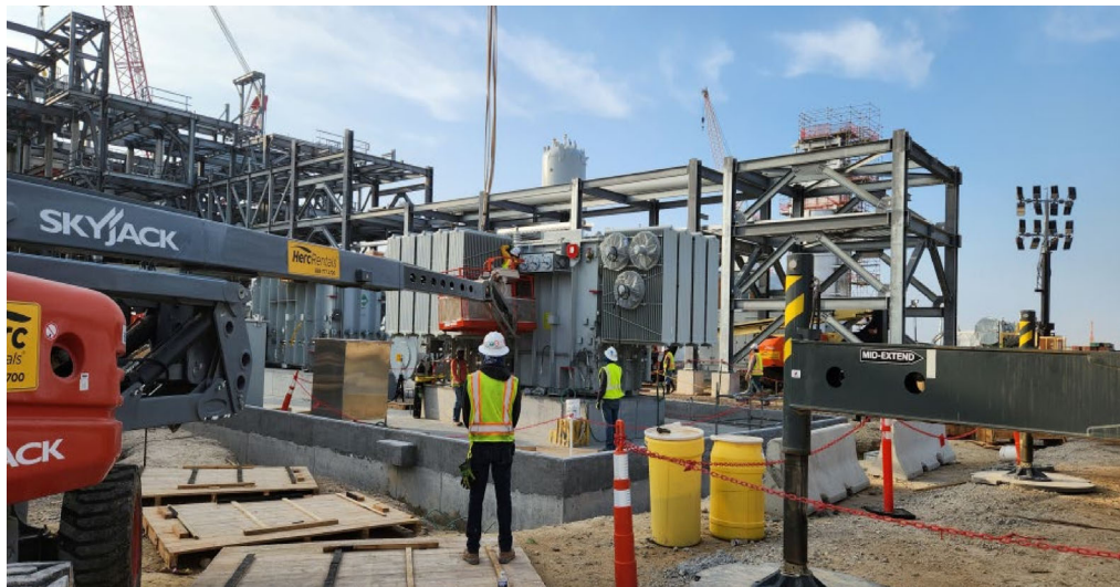
Photo 6: 311N01 Train 1 Liquefaction Main Transformer Set
