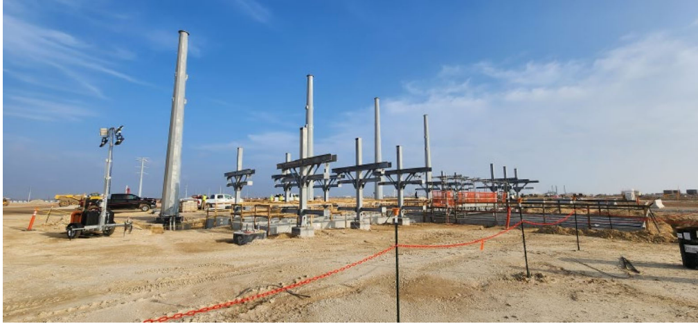
Photo 1: 310S01 OSBL Switchyard HV Poles & Supports
