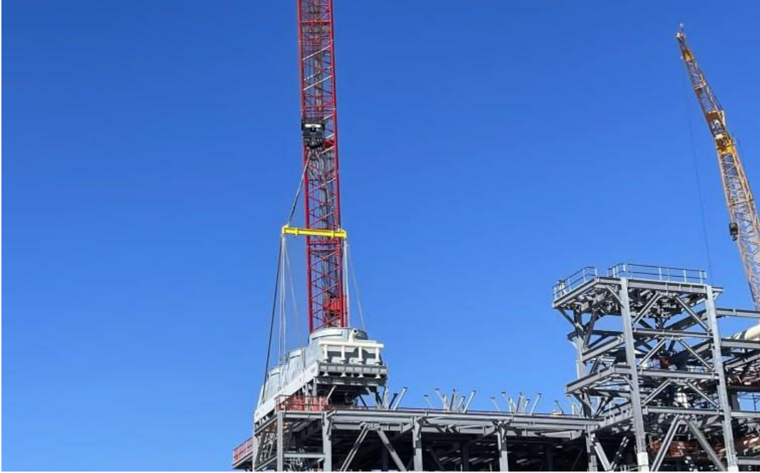
Photo 3: Area 311A01 Train 1 Air-Cooled Heat Exchangers
