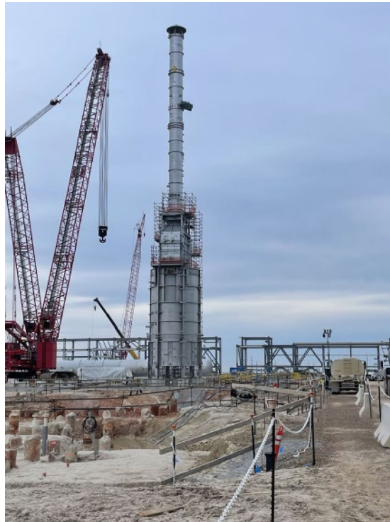
Photo 4: 322M01 Train 2 Hot Oil Furnace
