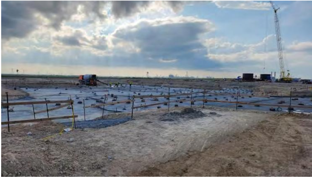
Photo 1: Area 310M01 Ground Flare 1 (OSBL East)
