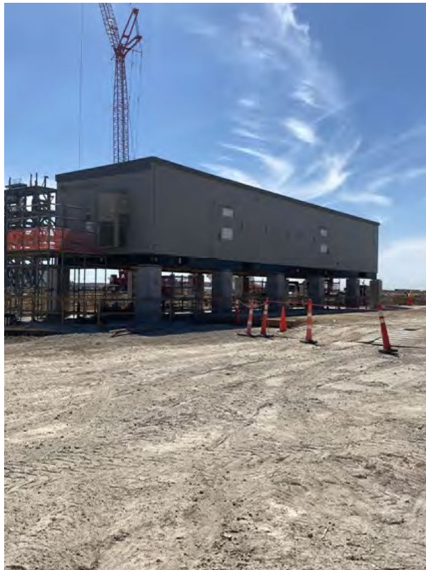
Photo 4: 333G01 Train 3 Utility Substation Set
