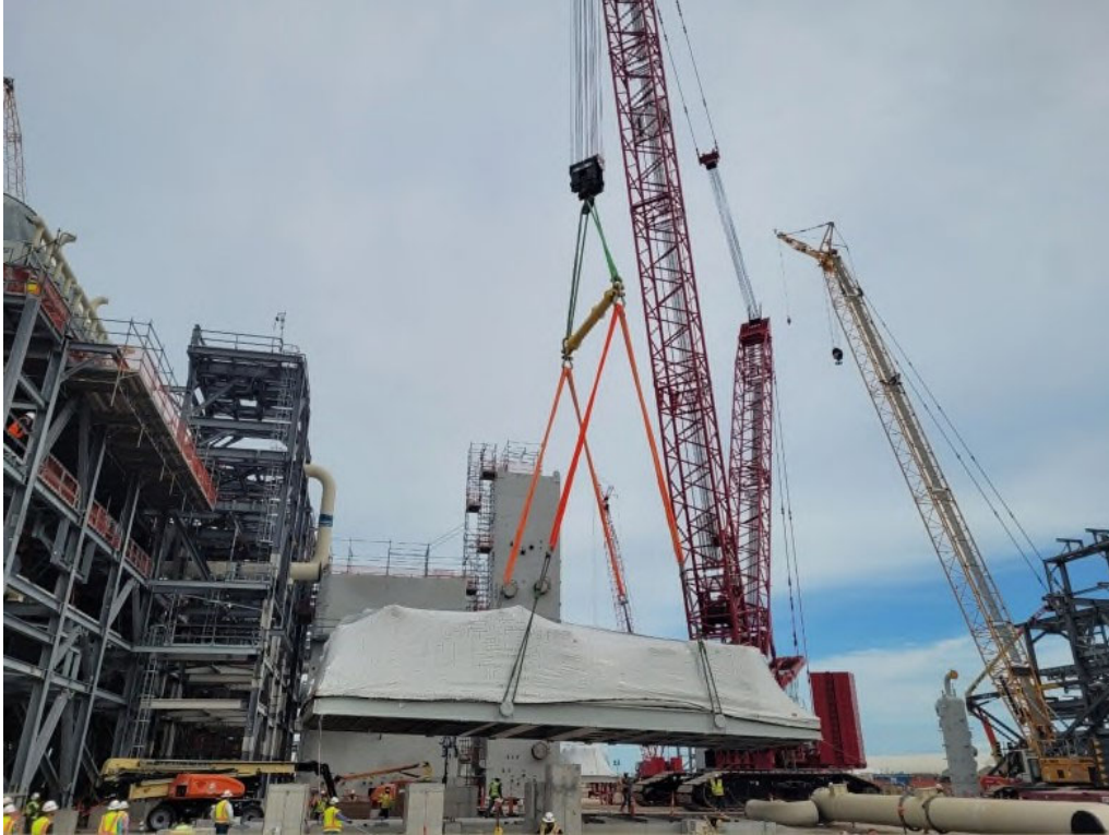
Photo 1: Area 311A01 Train 1 Mixed Refrigerant Compressor Set
