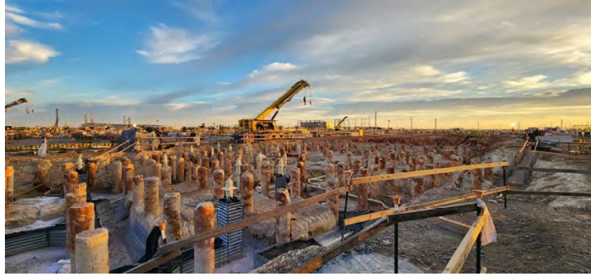
Photo 3: 333K01 Train 3 Underground Amine Pipe
