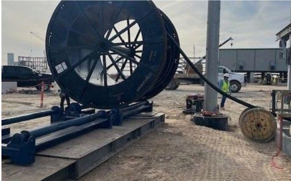
Photo 5: 310D01 3,000 KCMIL HV Cable Staging
