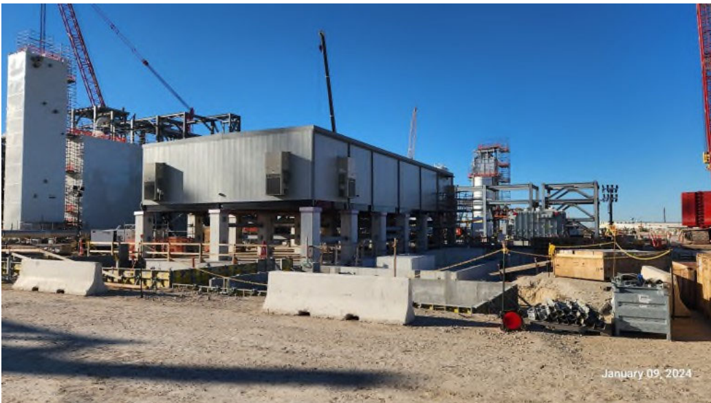
Photo 2: Area 311N01 Train 1 Liquefaction Substation Set
