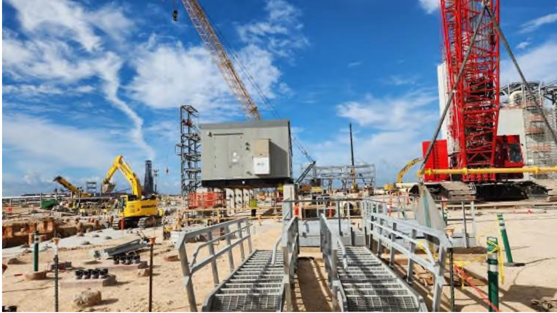
Photo 1: Area 311G01 Train 1 Utility Substation
