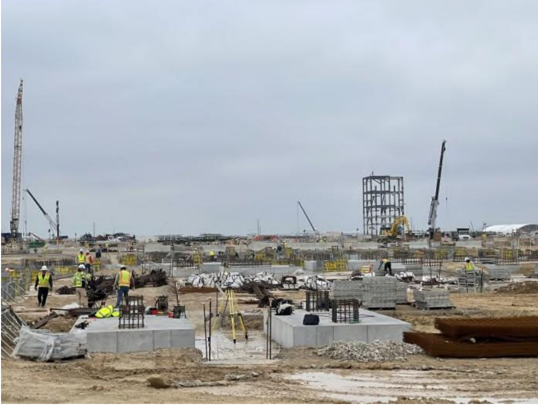
Photo 5: Area 310M01 OSBL East Ground Flare 1
