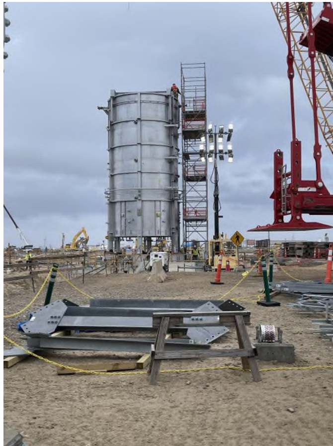
Photo 6: Area 322M01 Train 2 Hot Oil Furnace Assembly
