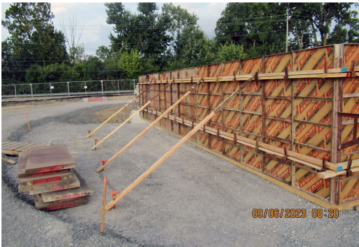
Phase 5 reconstruction included framing to add protective waterproof concrete around the top of the undisturbed low-level radiological waste entombment.
