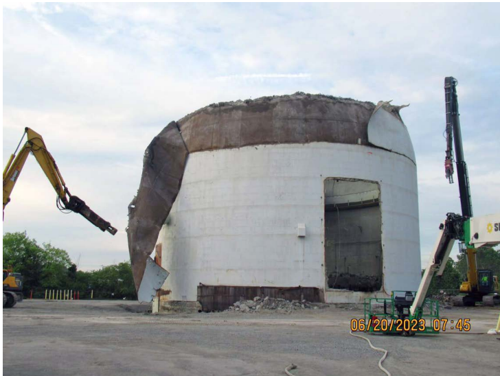
Phase 4 required elevated torch cutting the dome's steel skin, then "peeling" it away before demolishing the concrete reactor building from the top down.
