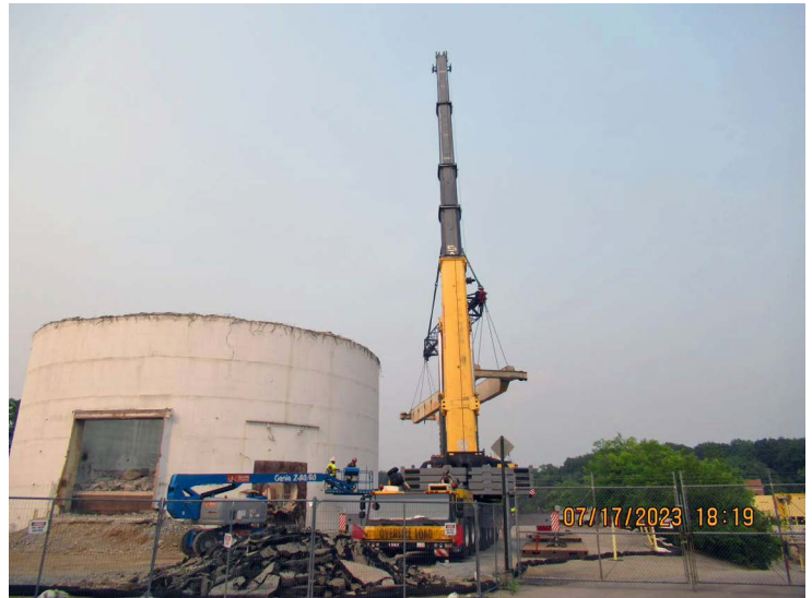
Phase 4 included a 30-ton crane safely removing the gantry bridge crane from inside the reactor building.
