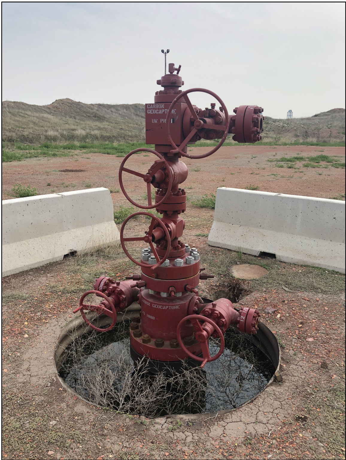
Source: Trihydro Corporation 2023. PRB Well 1 at DFS.
